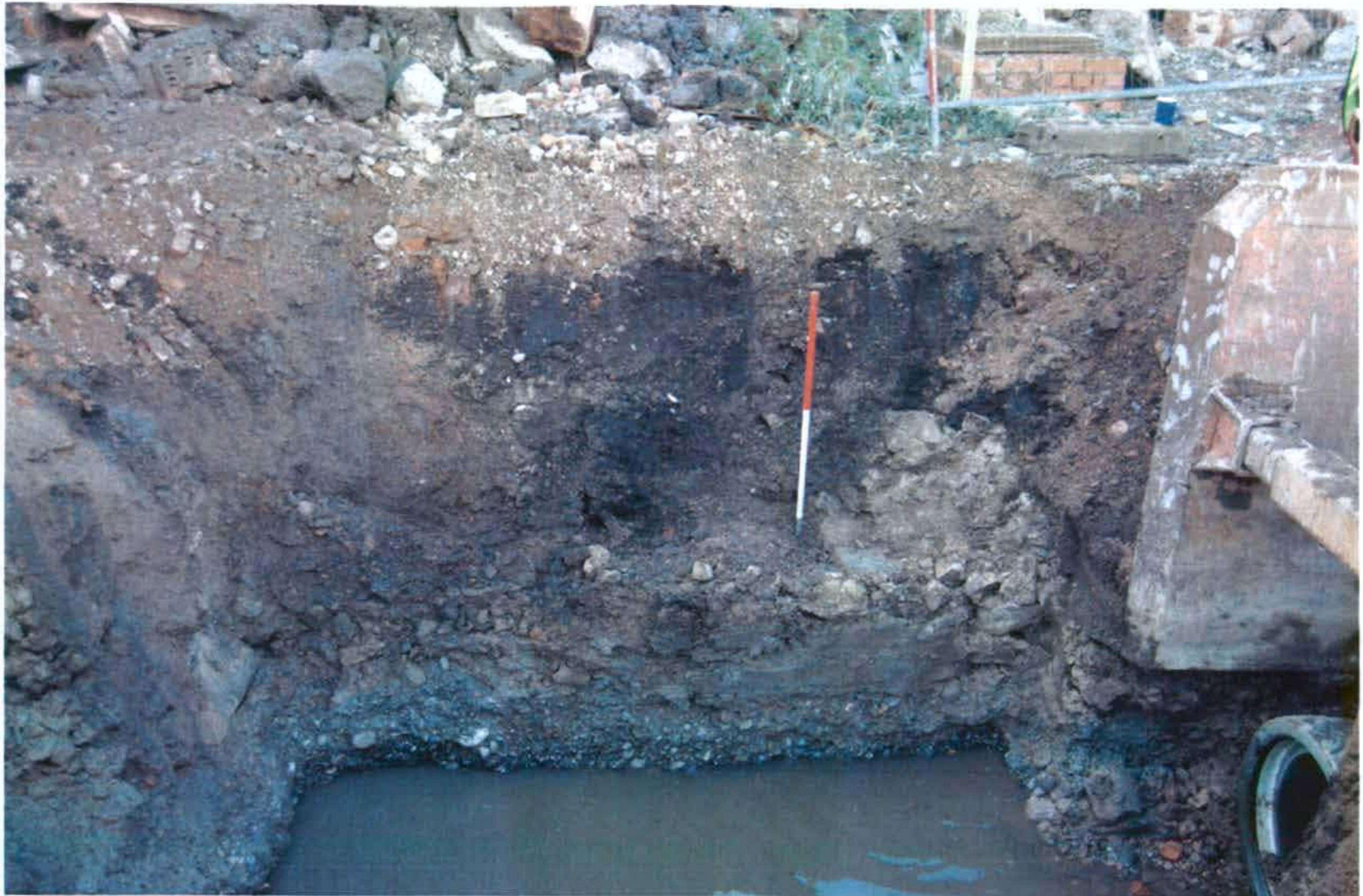
Fig. 9: Wall 6 visible in the intermediate manhole excavation. The base of cross wall 7 is also just visible as a single large stone on the left the photograph
