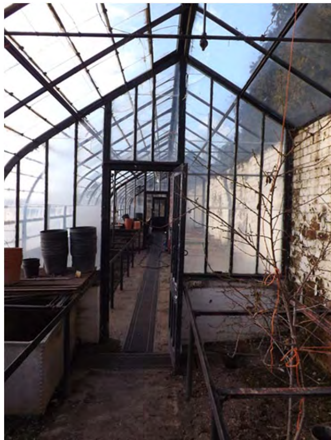
IBC 36: Interior of the greenhouse at a modular break. Note the heated/unheated sections and proprietary steel staging
