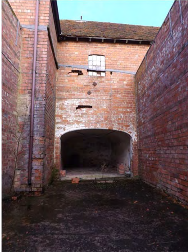
IBC 25: Beneath the garage, pig pens on the south, under-built in the hillside; upper windows are few, wasting the exceptional views
