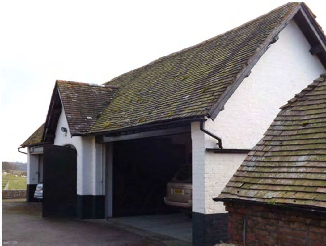
IBC 24: The garage, facing the house of Oversley Castle to the north
