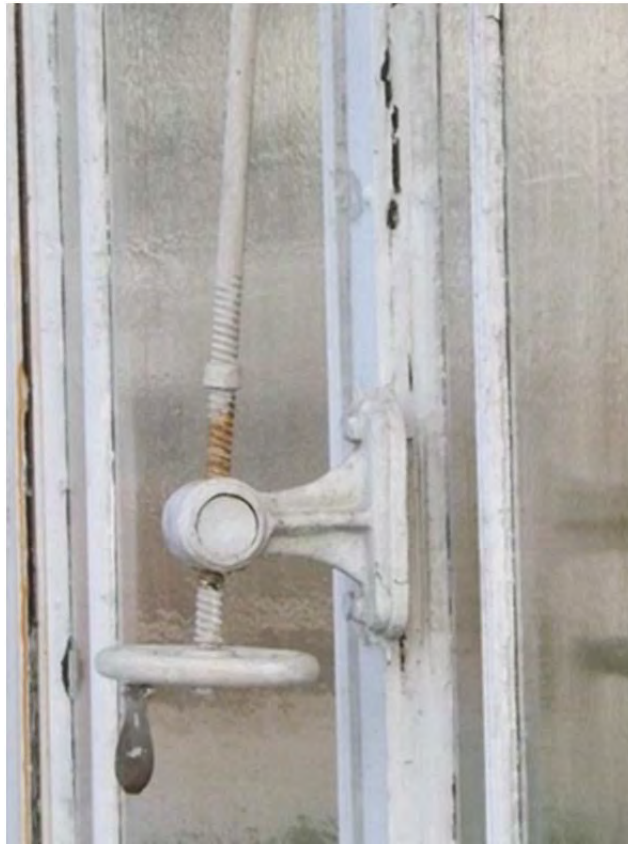
IBC 42: The louvre-crank ventilator system, common to both pool-house annexe and greenhouse
