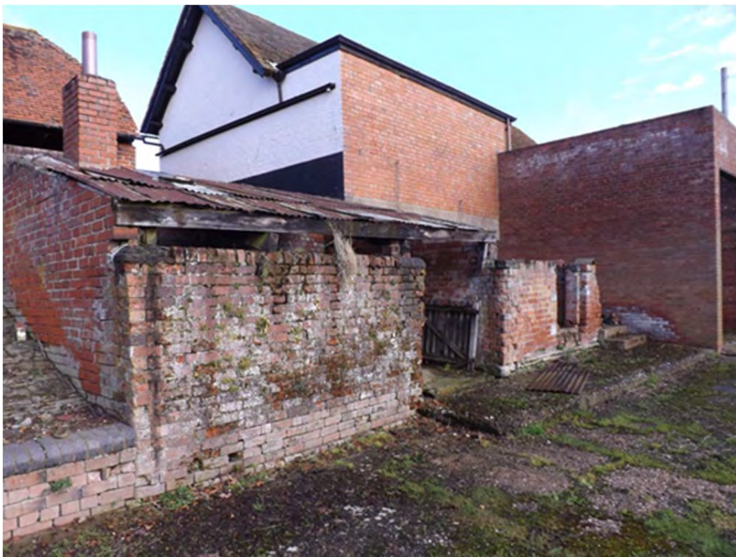
IBC 22: The forge, two distinct phases of side-wall; later baffle wall across front
