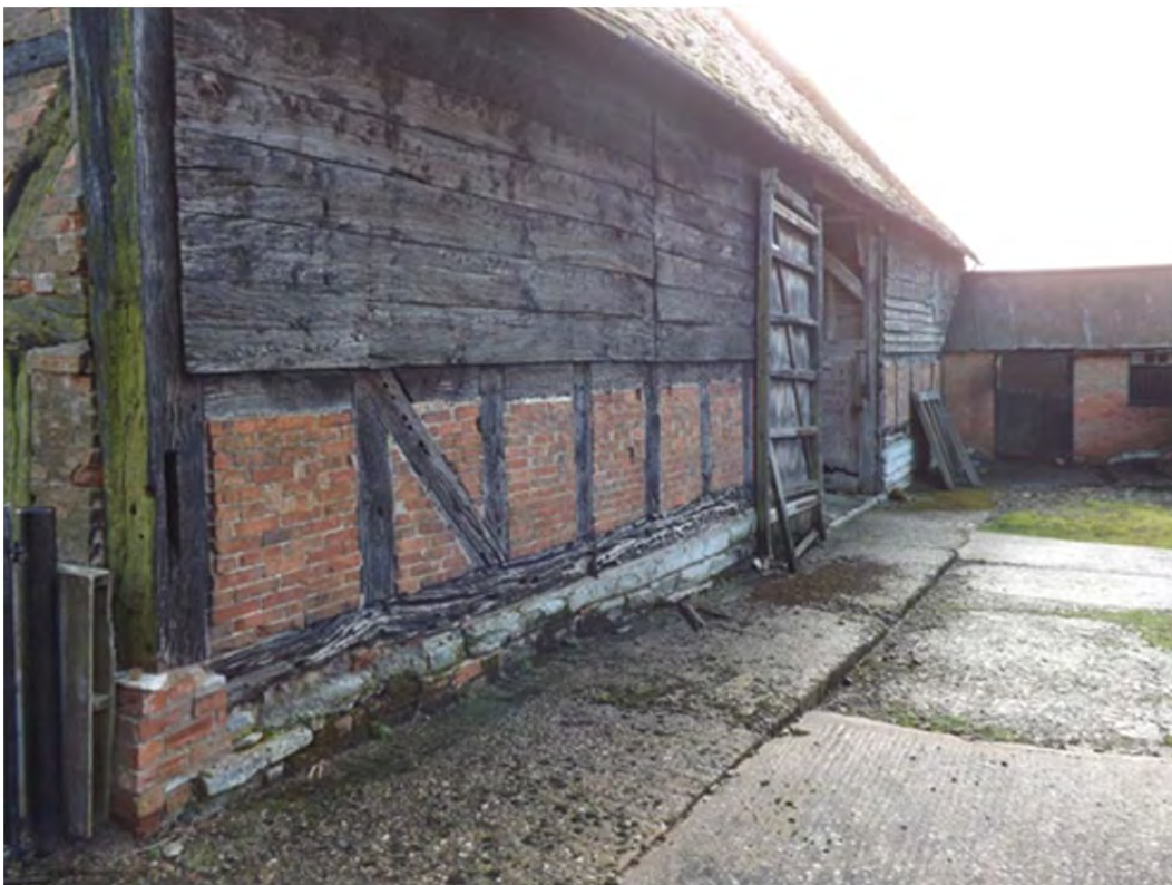
IBC 18: Barn exterior, plinth, box-framing, nogging and boarding. Note re-used corner post
