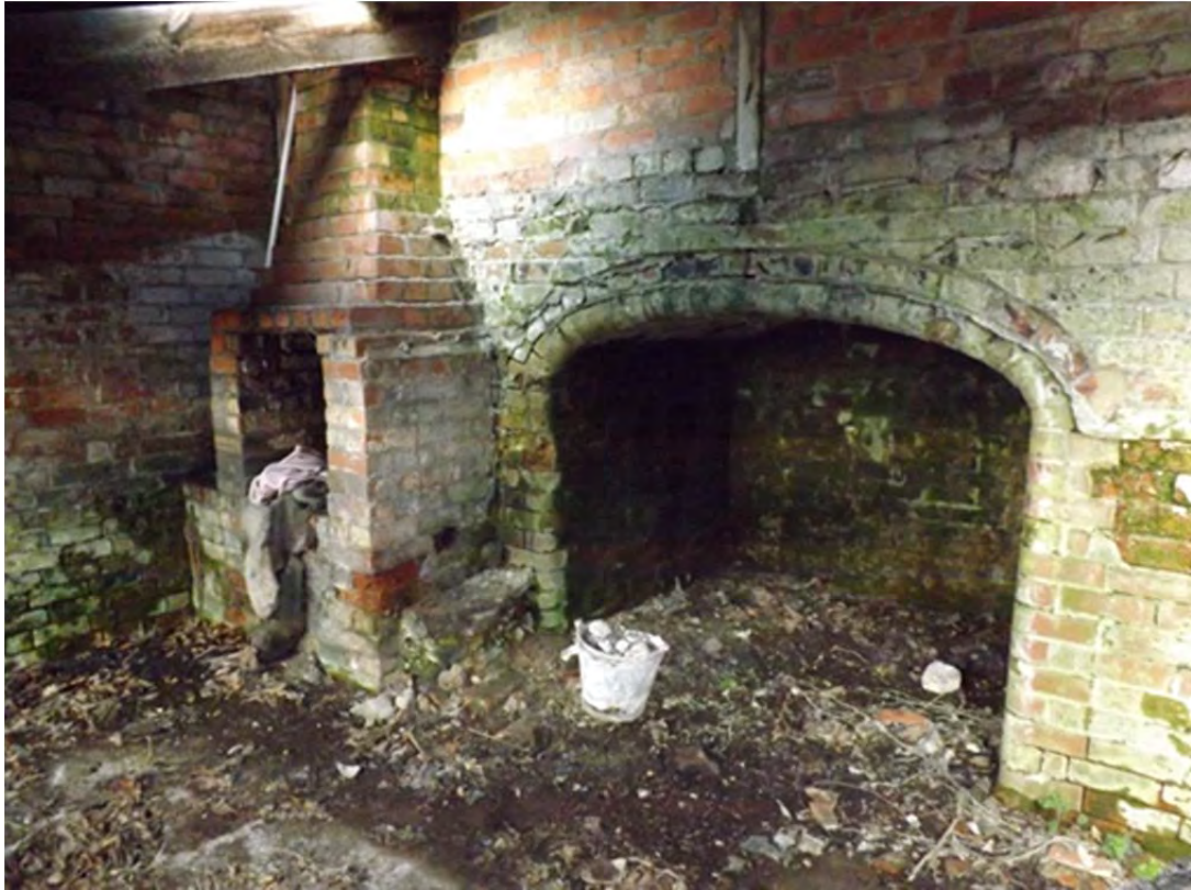
IBC 23: Forge interior: the hearth and alcove; two phases of side and rear wall distinct
