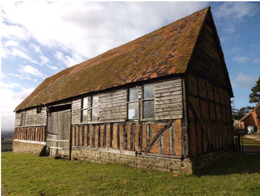
IBC 14: Barn exterior; east face - plinth, close-studding and boarding; gable – plinth, close studding, box-framing and boarded upper portion
