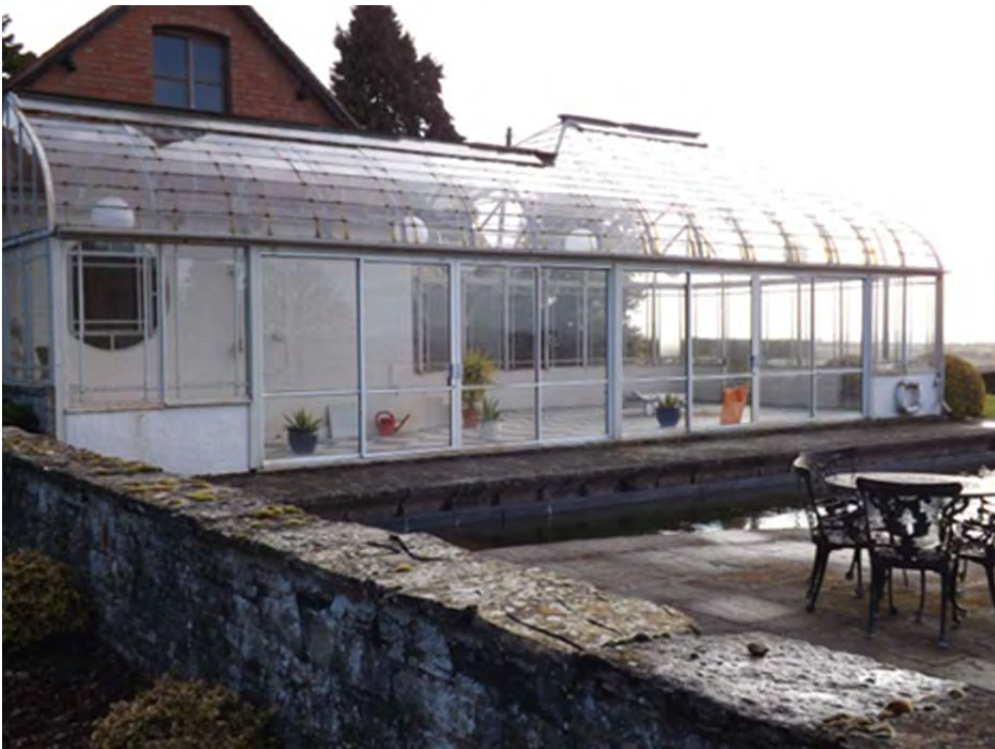
IBC 38: Pool house annexe, long, (west) face, half of its length replacement UPVC doors
