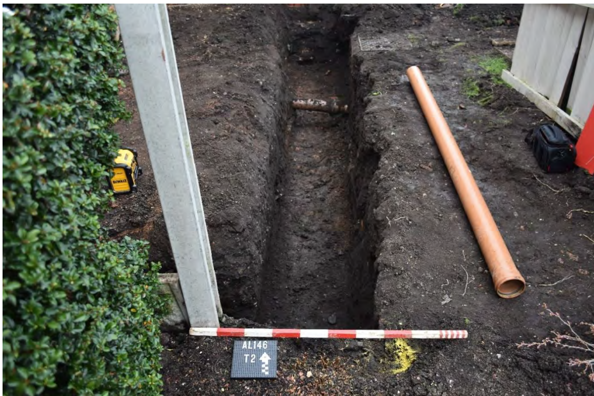
2: Trench on east side of the site, looking north, showing natural (2) at north end
