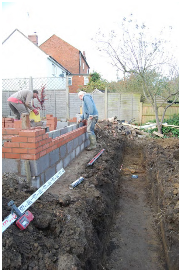
Fig 8: Boundary wall foundation trench looking north. Myrtle Cottage is the white house in the background
