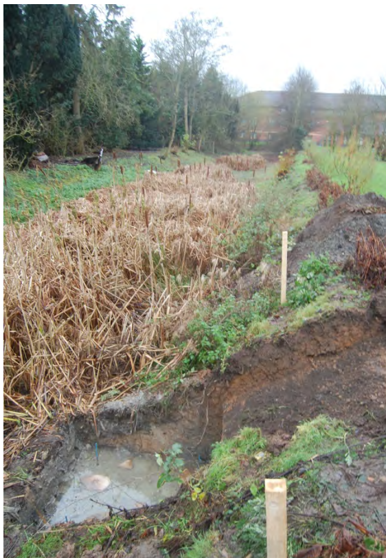
Fig 16: New service trench cutting across the line of the 17th century ornamental canal
