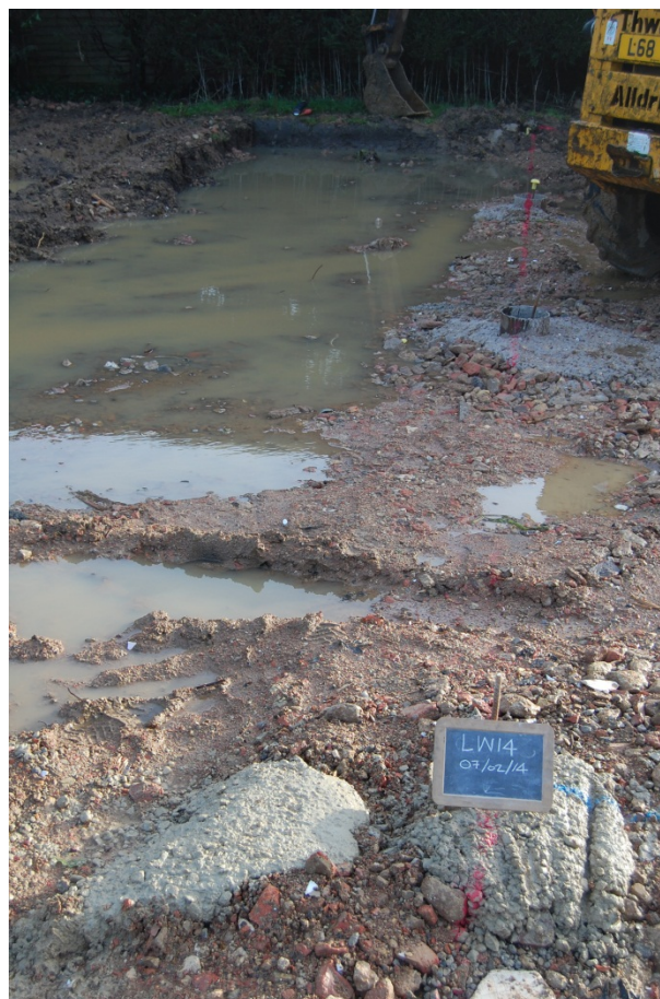
Fig 4: Ground water on site
