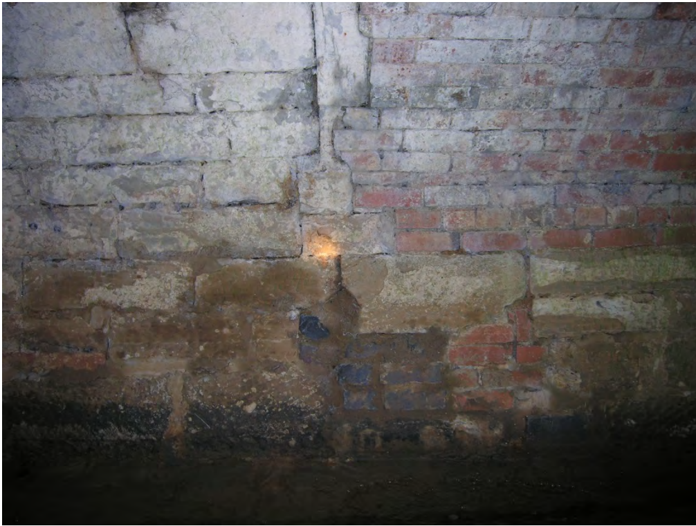
Fig 4: Original phase of bridge (left) with extension (right) and repairs below
