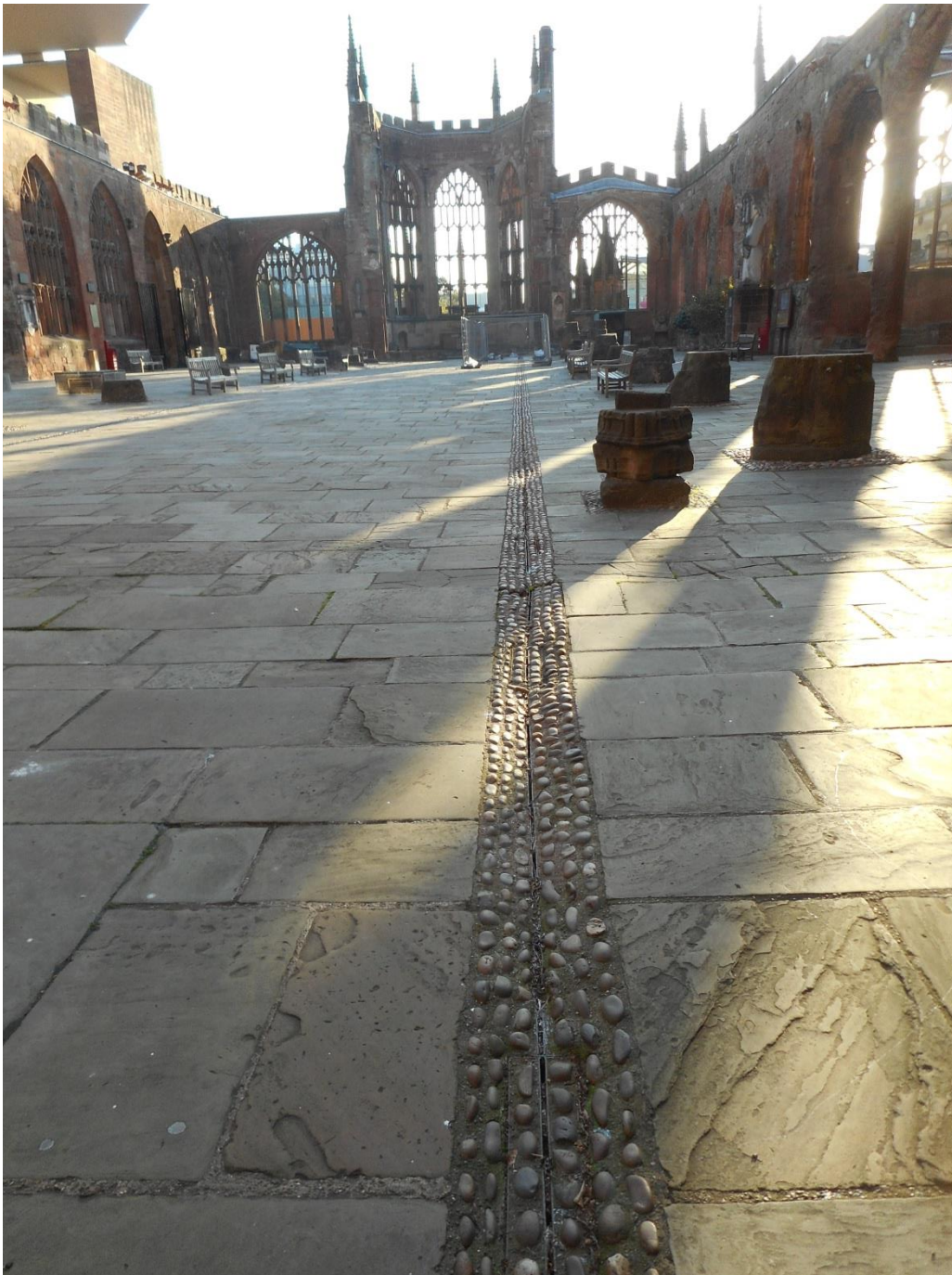
1: Slot drain prior to replacement
