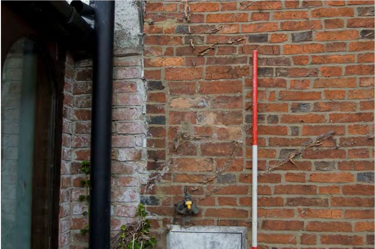
Fig 12: Blocked window in rear wall
