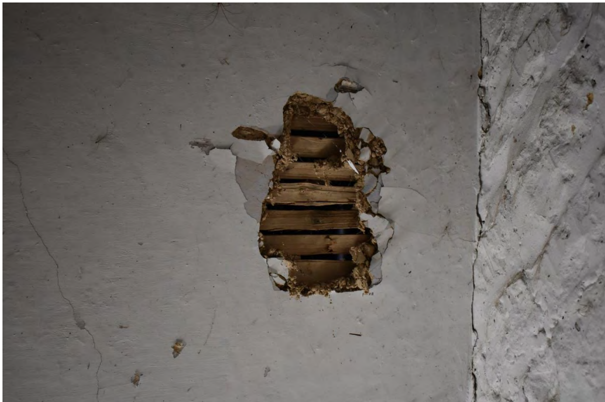
6: Plaster ceiling with laths exposed
