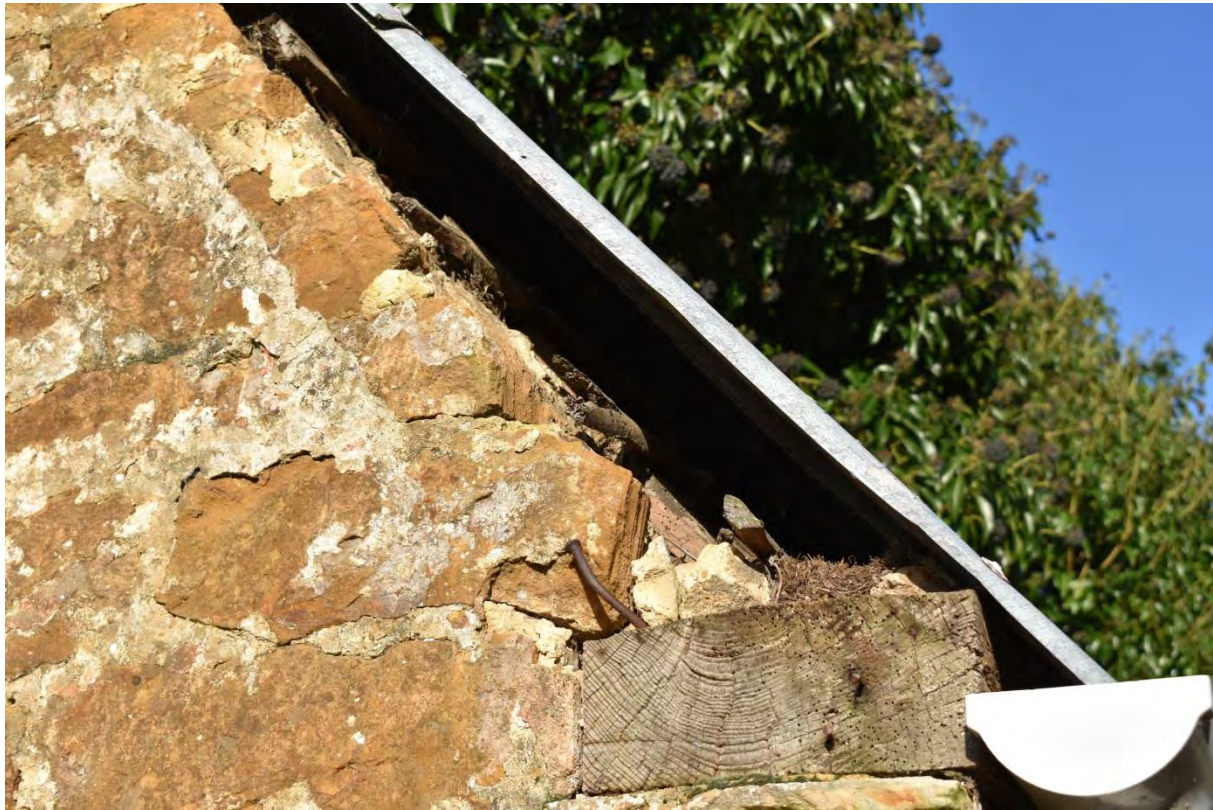
5: Old roof laths below corrugated iron
