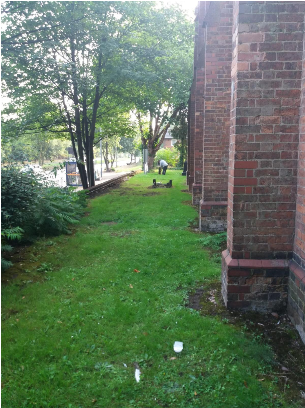
1: Area north of the church where drain was blocked
