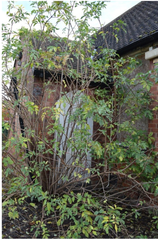
Photograph 4: Front door (blocked)
