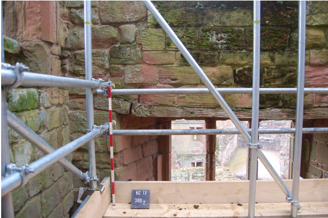
37 NW room, top floor, lintel (Drawing 37, Sheet 10/4) HE sample 3
