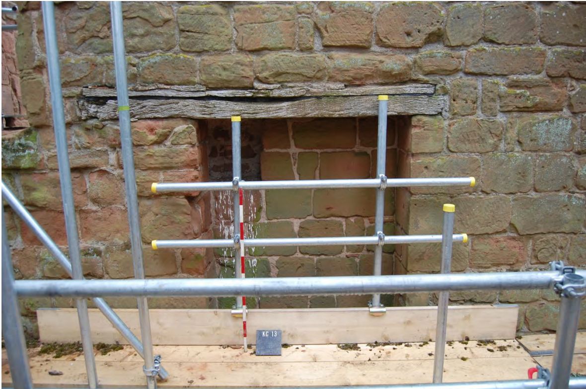
39 NW room, top floor, lintel (Drawing 40, Sheet 12/1) HE sample 1
