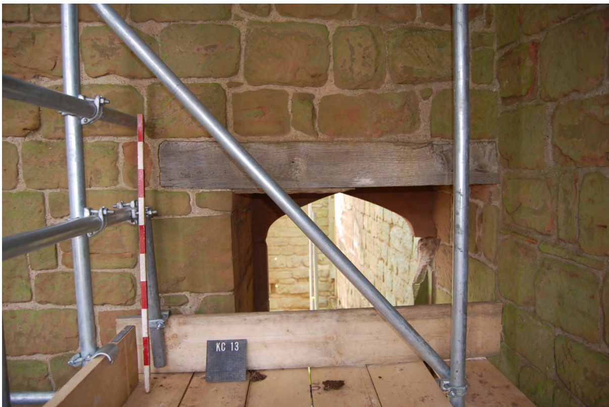
38 NW room, principal floor, lintel (Drawing 38, Sheet 11/1) HE samples 5, 24, 25, S room, top floor, Drawing 39 (Sheet 11/2) is of a concrete lintel and was not photographed
