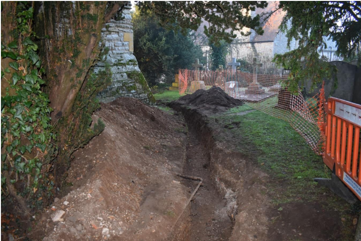
3: Service trench for water main on the north side of the church
