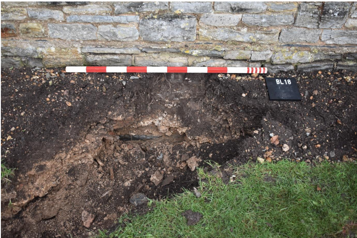
6: South aisle wall with layer of degraded building material 102
