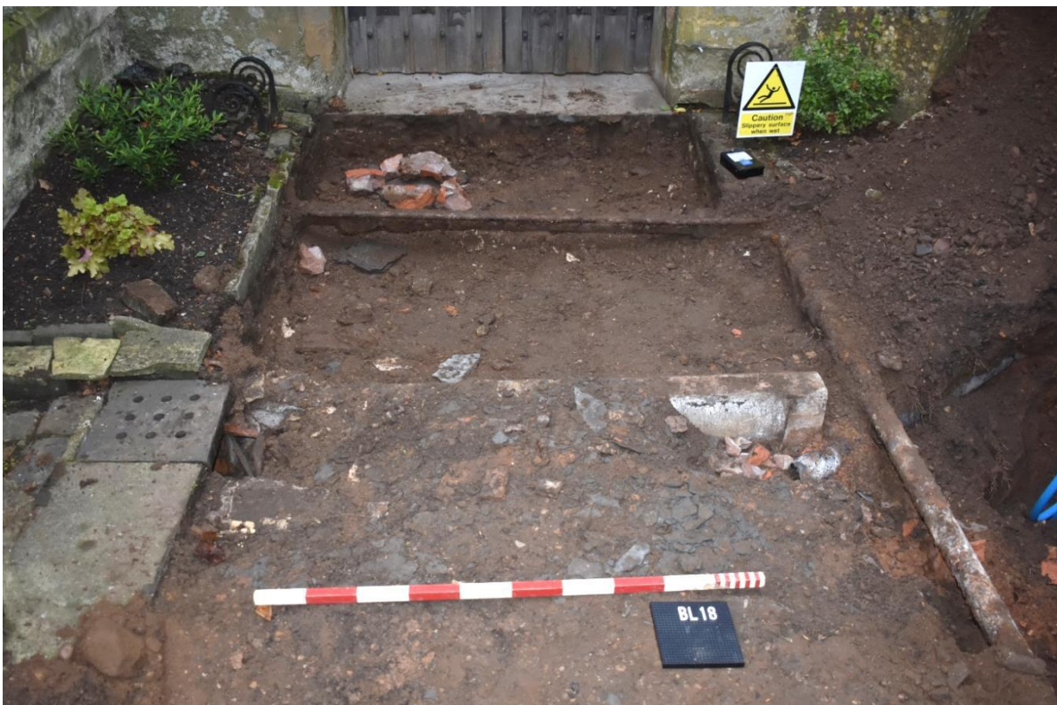
4: Area in front of north door, where slabs 105, were lifted, exposing the reddish brown layer 104, and the concrete casing for soakaway 107
