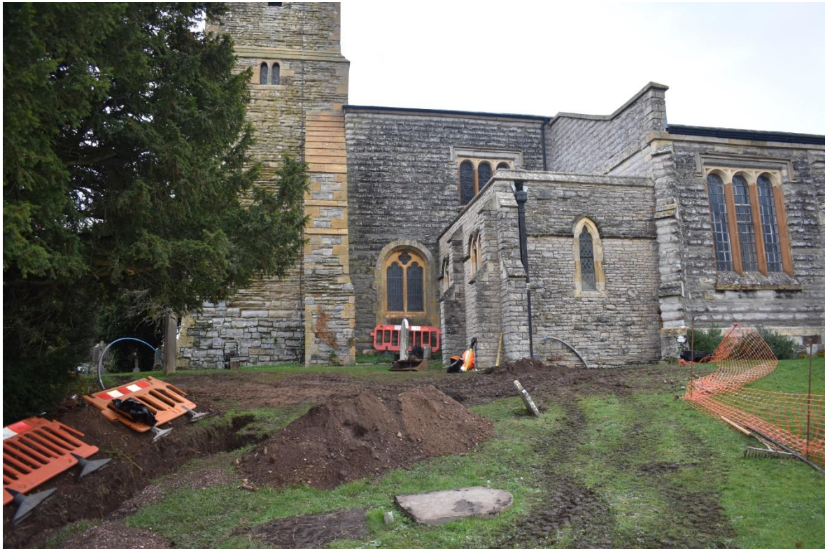
1: Service trench for waste water excavated from the river to the south side of the choir vestry
