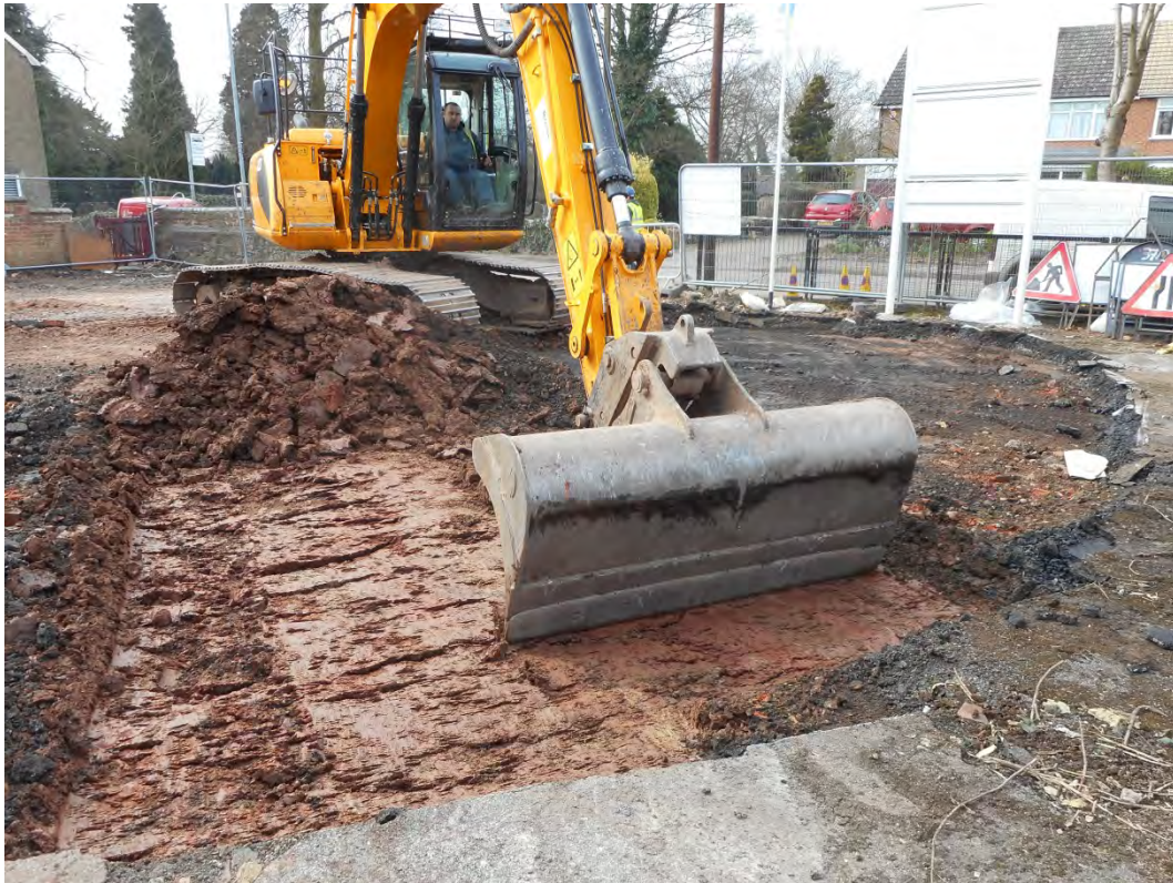
1: Disturbance to front of site, looking SW
