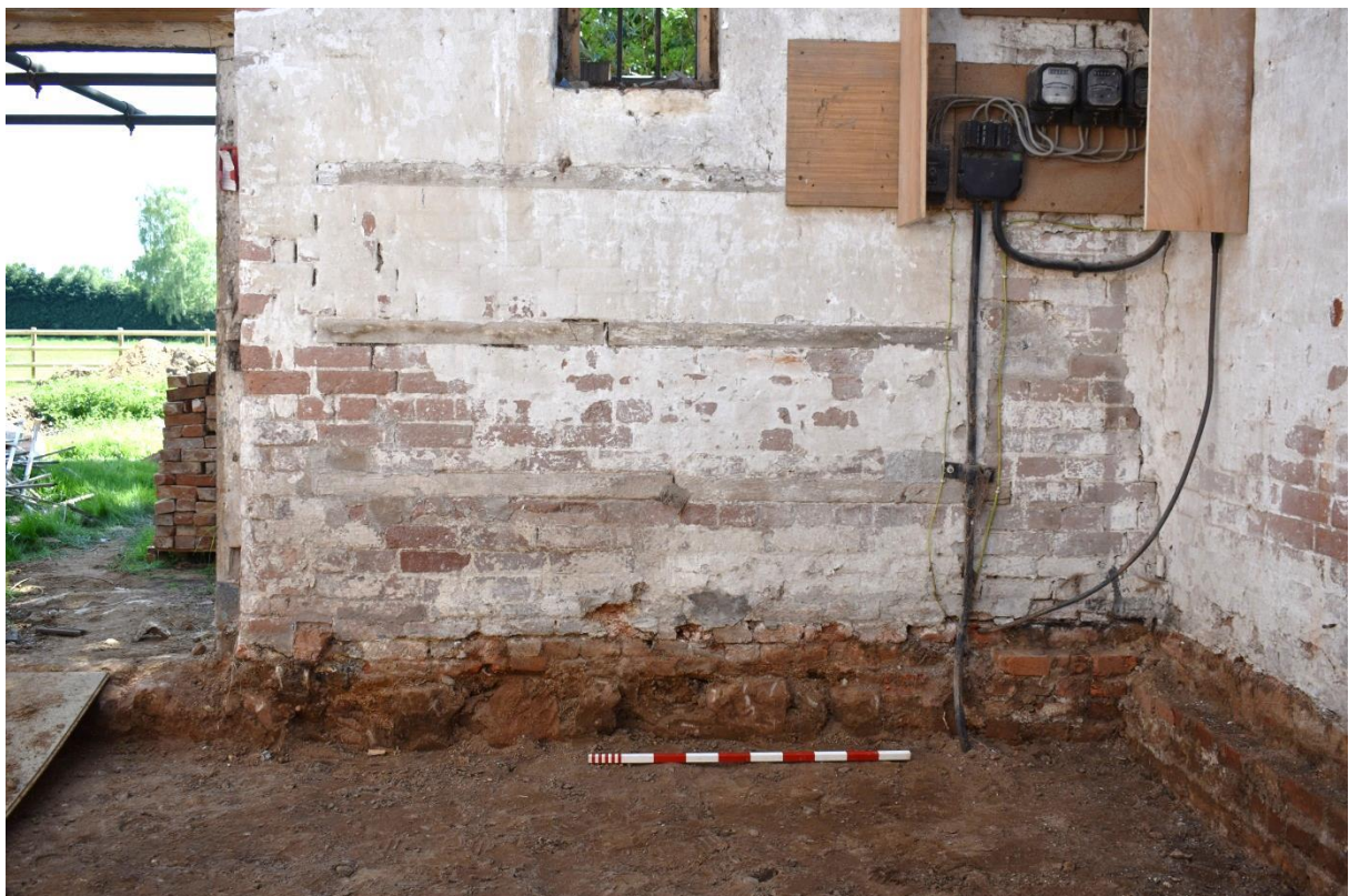
54: Stone footings to south wall and offset brick footings of re-built gable wall
