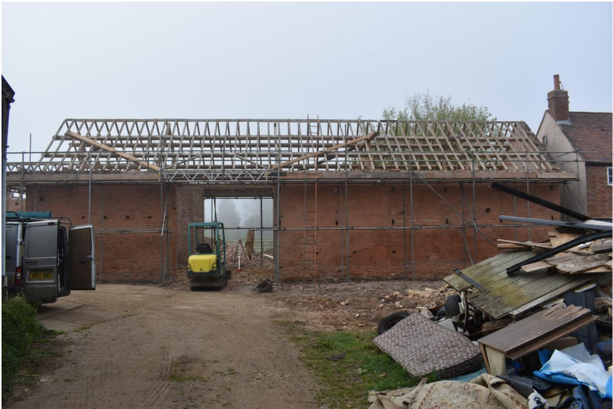
61: The barn and cow house with roof tiles removed and lean-to demolished
