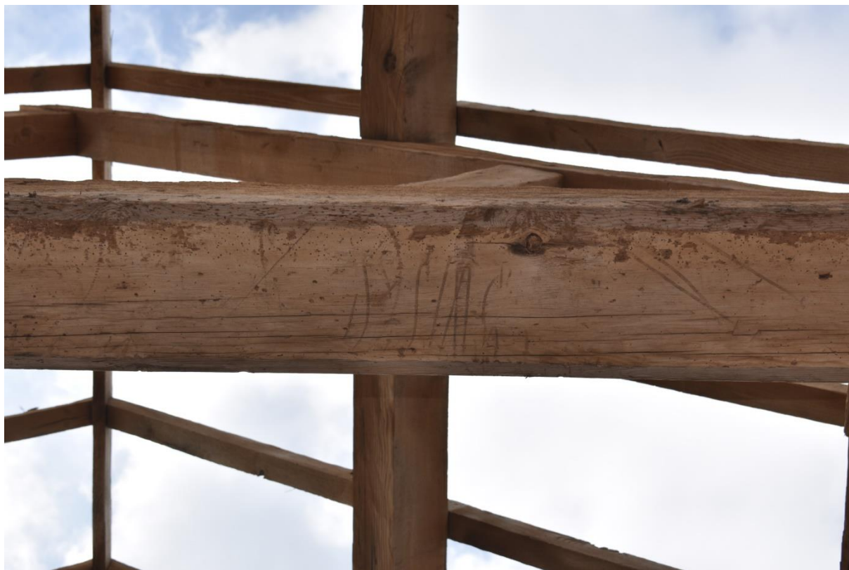
63: Incised marks on underside of one of the tie beams
