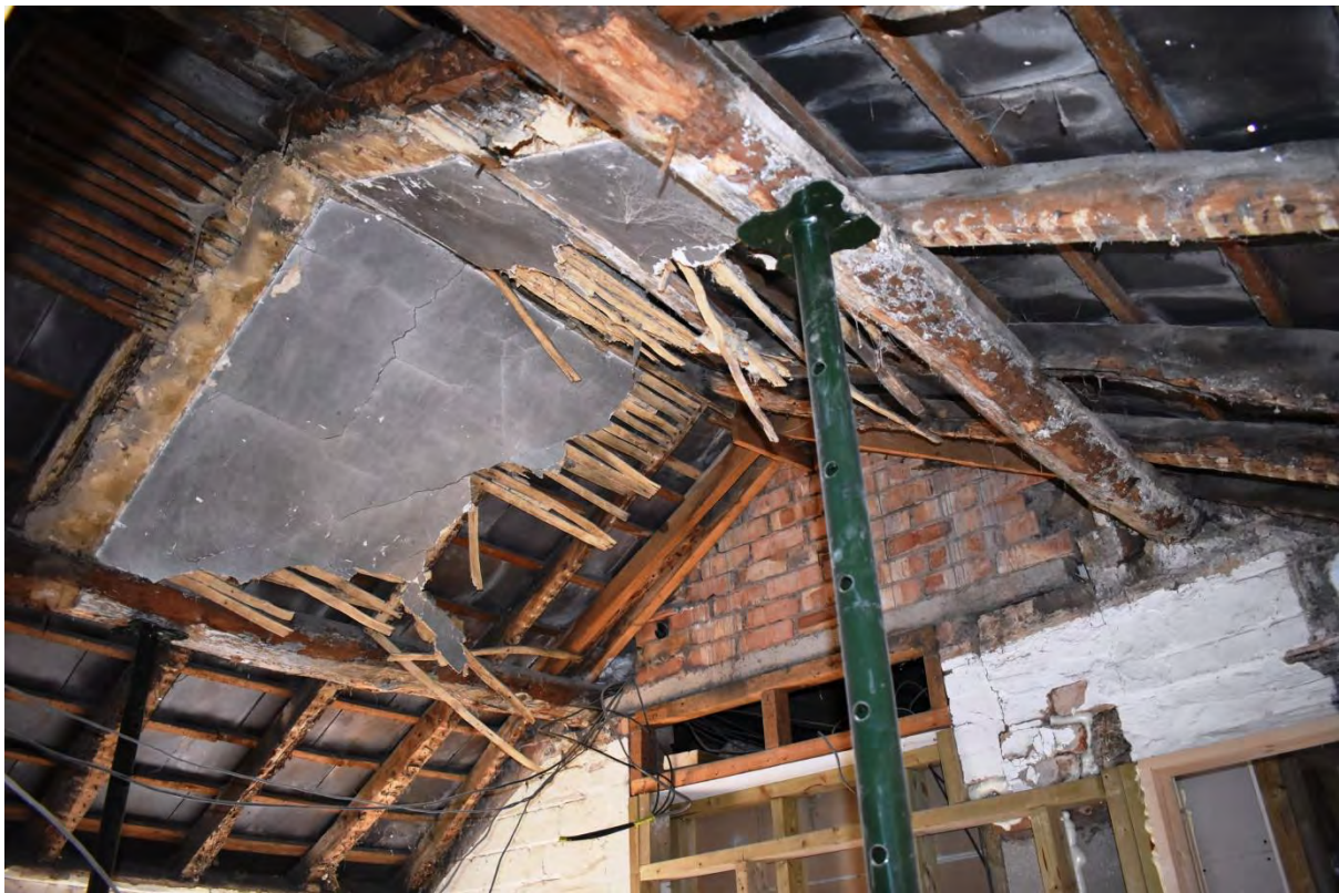
18: Last surviving fragment of the original lath and plaster ceiling in the stables
