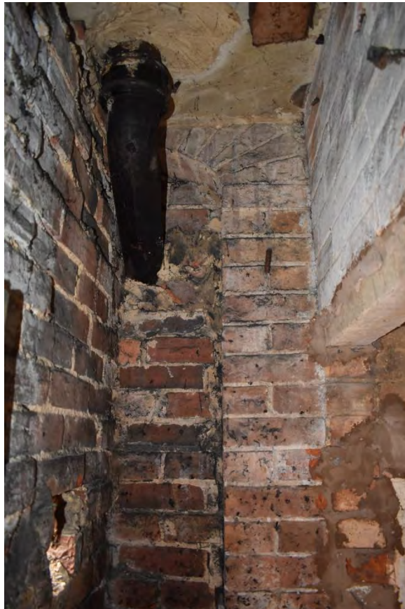
9: Addition to rear of adjacent building encroaching into archway
