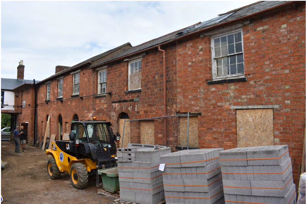
3: General view of the front of the stables with the three phases visible as changes in the roof height and the bricks used
