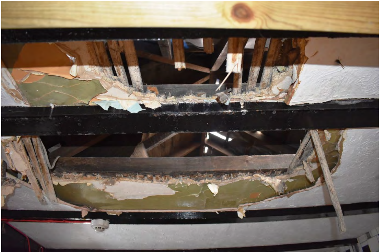
13: The ceiling in the bar (Room 1) during demolition showing the original lath and plaster ceiling that was replaced by modern plasterboard and fake beams
