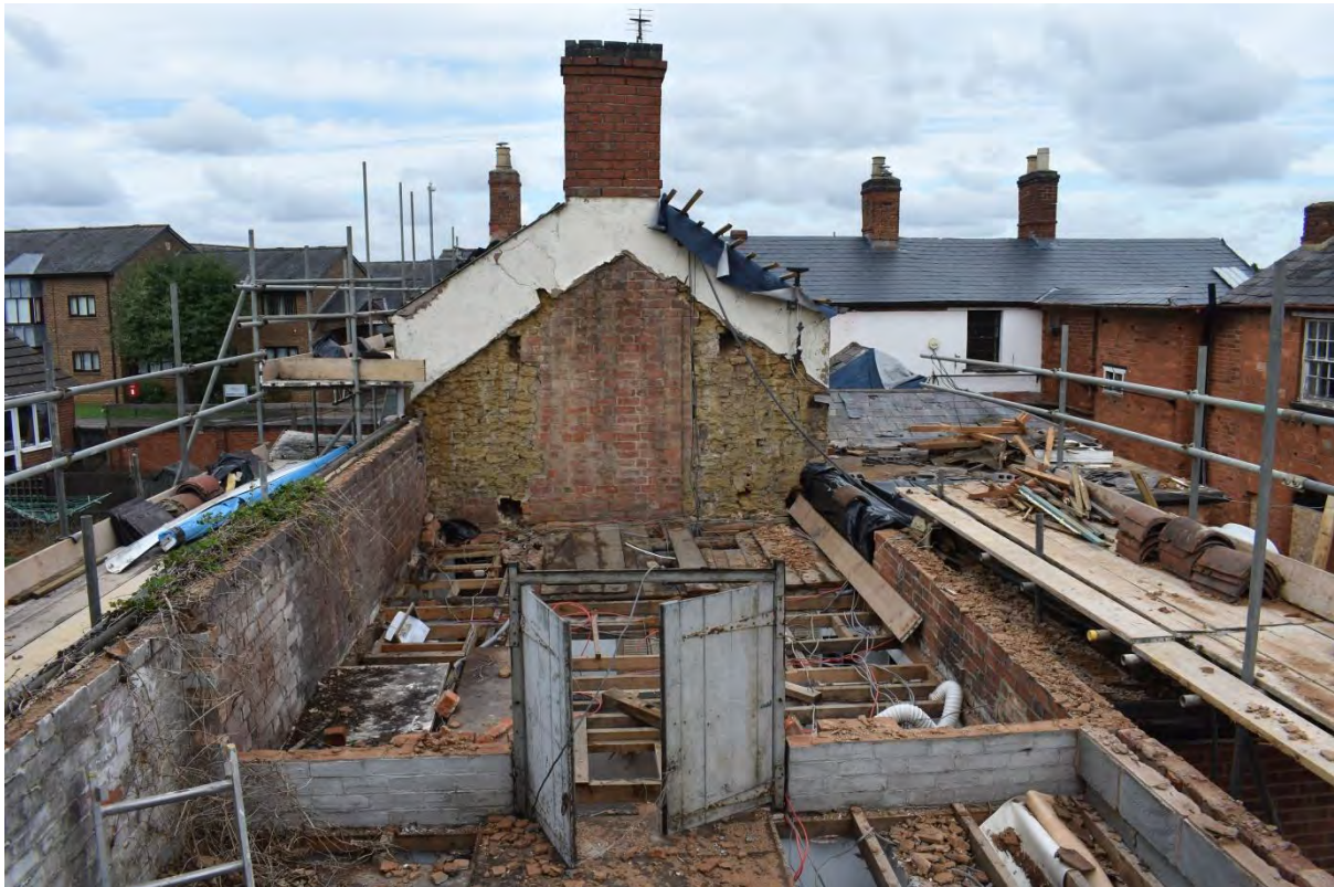
8: The brick chimney for the fireplace and ovens in ground-floor Room 2 and the partial demolition of the south-east extension
