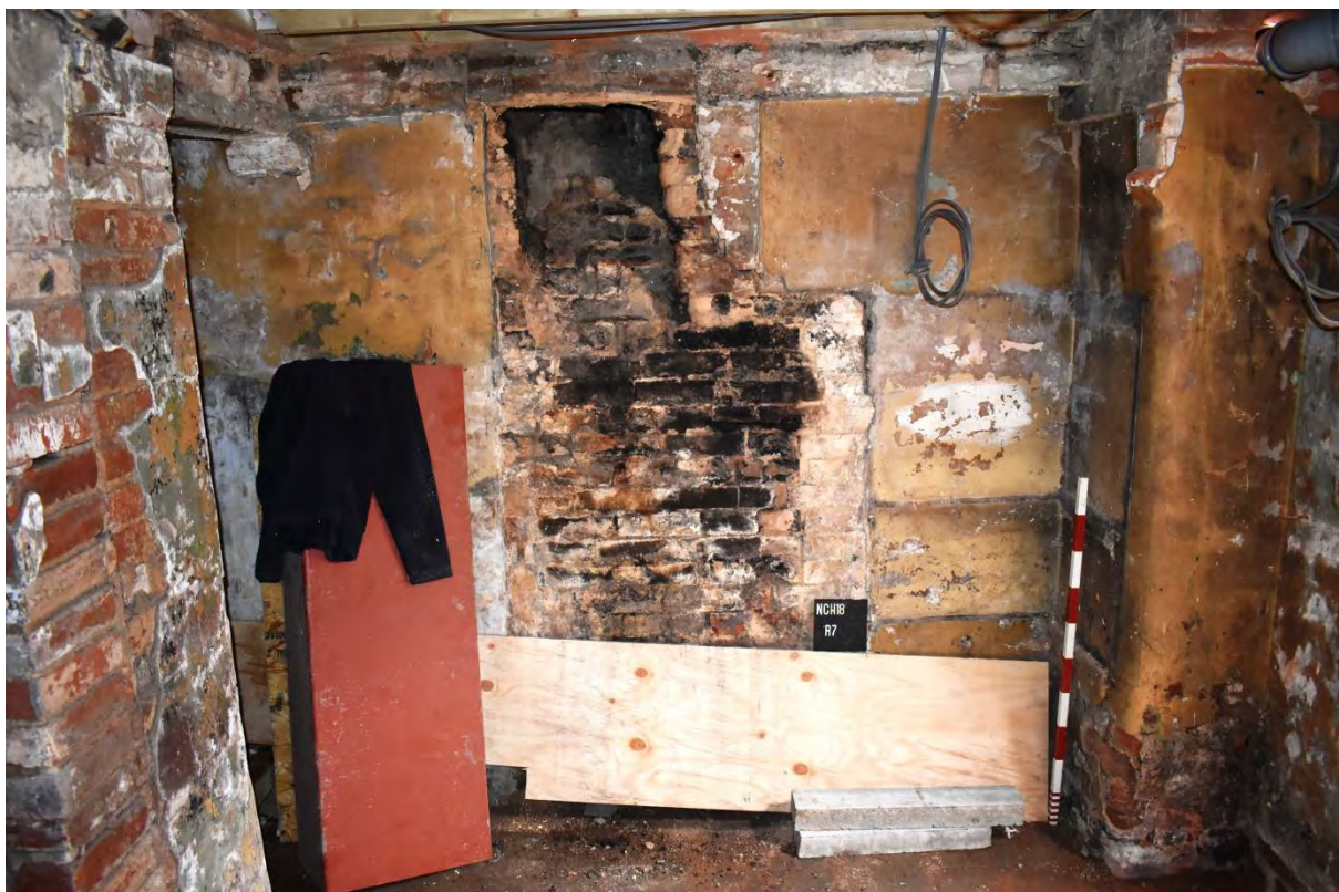
22: The north-east wall of Room 7 showing the chimney from the removed fireplace
