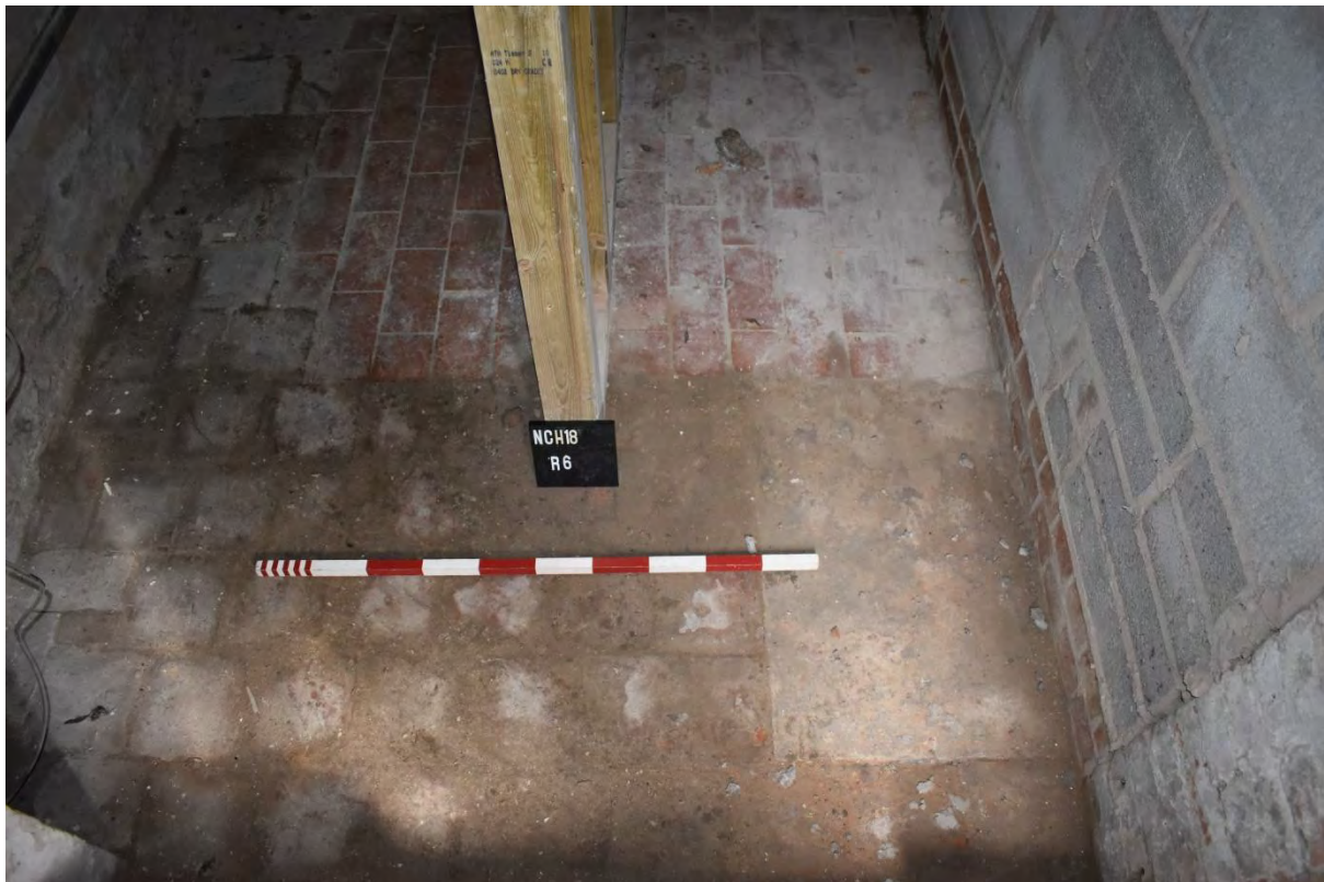
21: Brick and tiled floor of Room 6 and new internal walls added for this renovation
