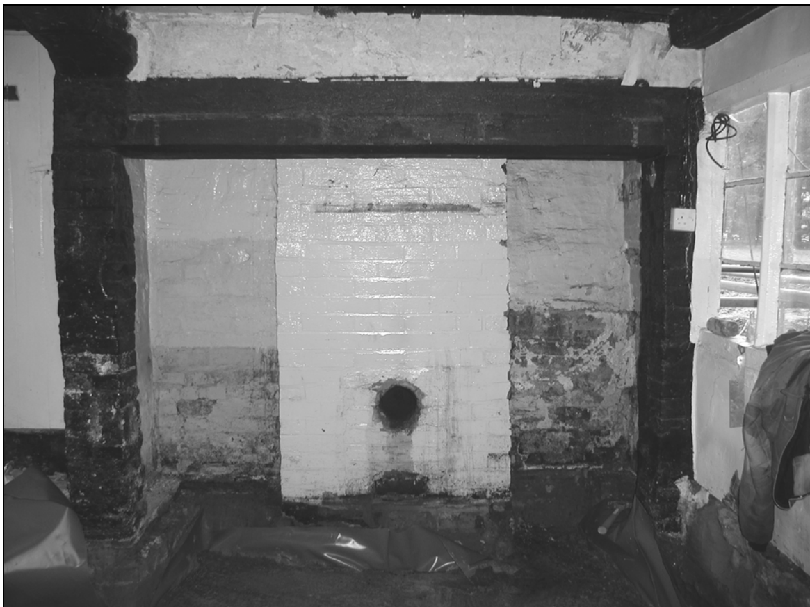
Fig 7: Fireplace with inserted brick flue
