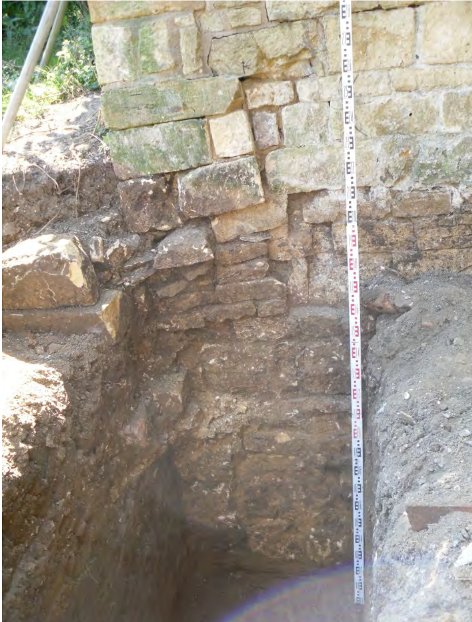
Fig 30: The interior of the far eastern end of the standing garden wall as exposed in new foundation trench. It shows the wall's deep foundations and partial collapse towards east
