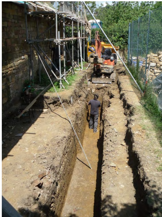
Fig 29: Foundation trench on the east side of Coach House, viewed from the northwest
