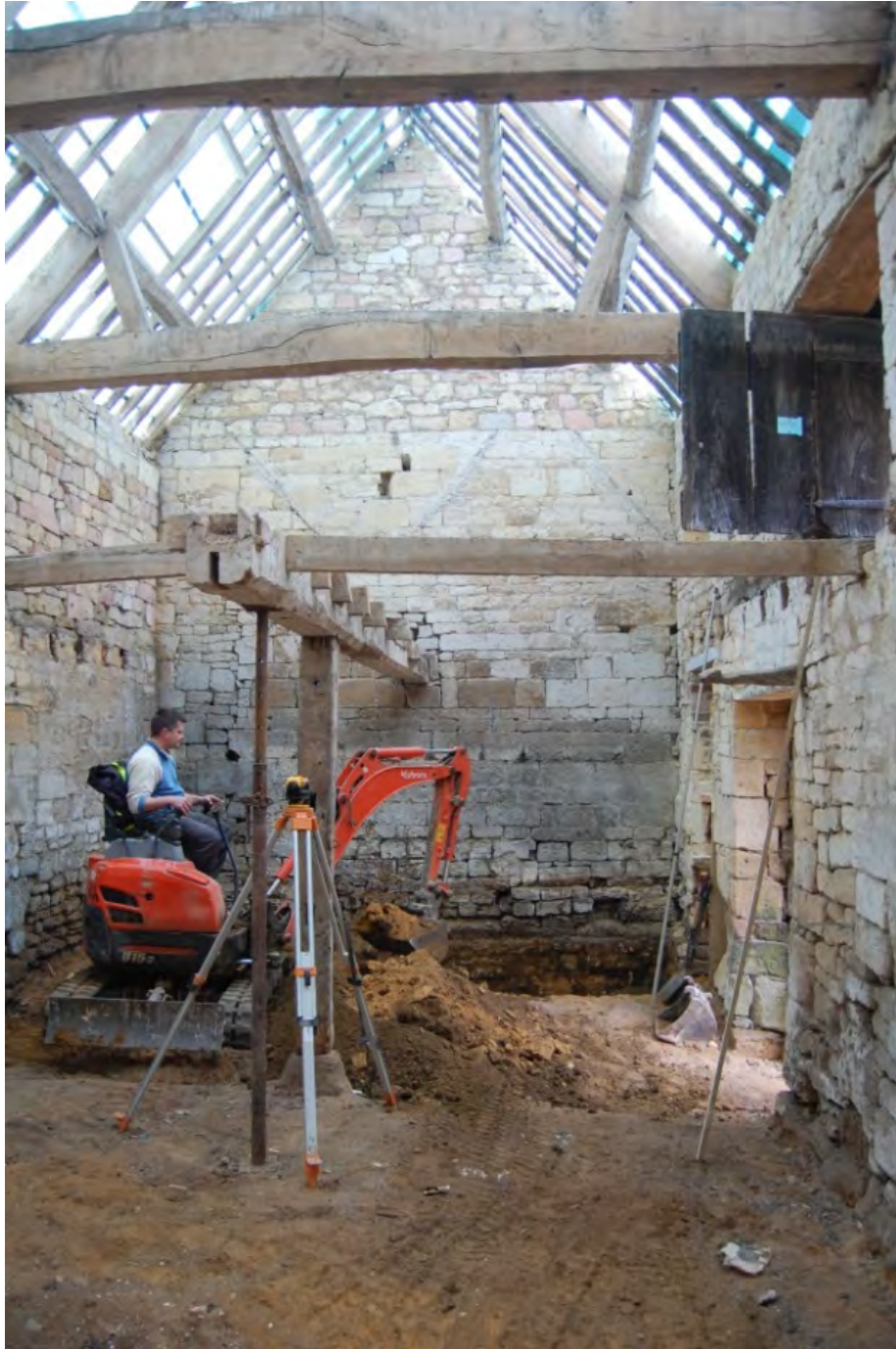
Fig 16: The interior of the south gable in Room B. The original garden wall can be seen (large yellow stones) with the gable added to the top. The double roof scar of a building shown on early engravings can also be seen. The ground level is in the process of being reduced. Burnt stone can be seen in the east and west walls of the building and in the top part of the gable but not in the older garden wall
