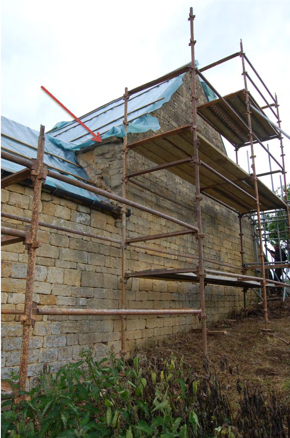
Fig 9: The exterior of the south gable of Room B. The wall scar (arrowed) shows that the original garden wall which forms the lower part of the gable, once continued at this height, at least to the west, and probably continued at this level across the top of the gateway
