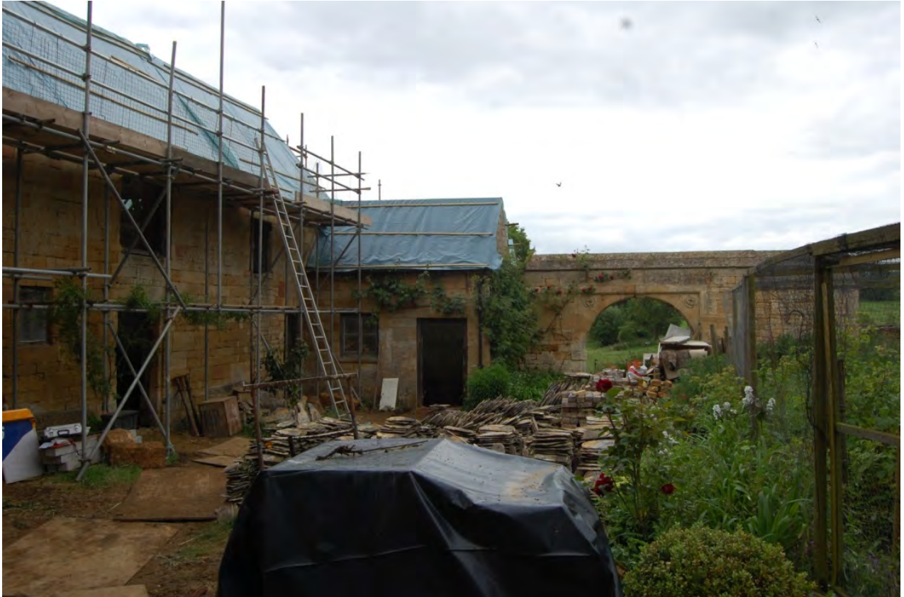
Fig 5: General view of the of the courtyard containing Coach House (left) looking south
