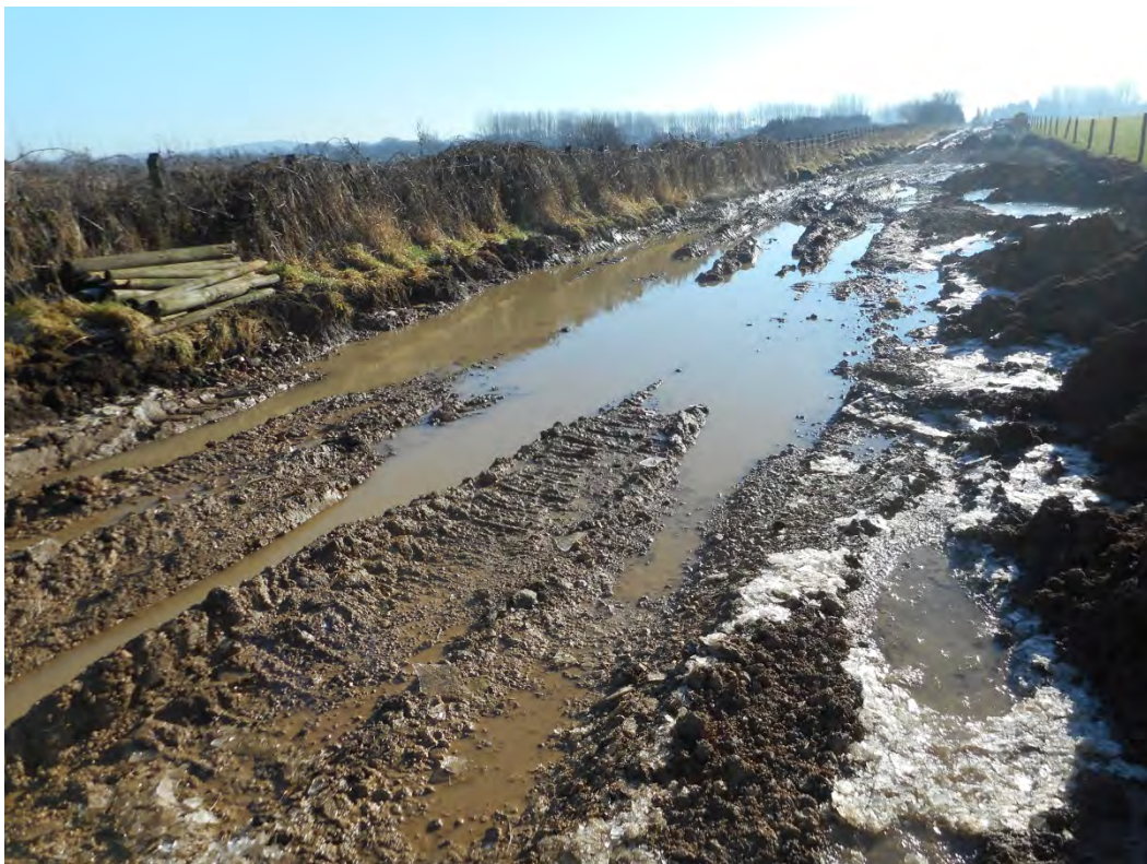
2. Waterlogged stripped area, middle of embankment strip, looking south
