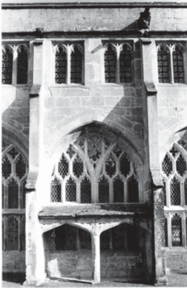
Fig. 333 Cloister bay 4, after restoration and glazing in the late 1980s, showing the northern pentice (Structure 19B)
