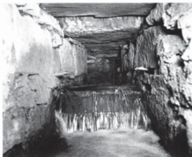
Fig. 394 View east inside Bekynton's conduit of c. 1451, adjacent to the Camery wall. The weir was created when the water level was raised in St Andrew's Well, probably in the early nineteenth century. The floor of the conduit was also raised
