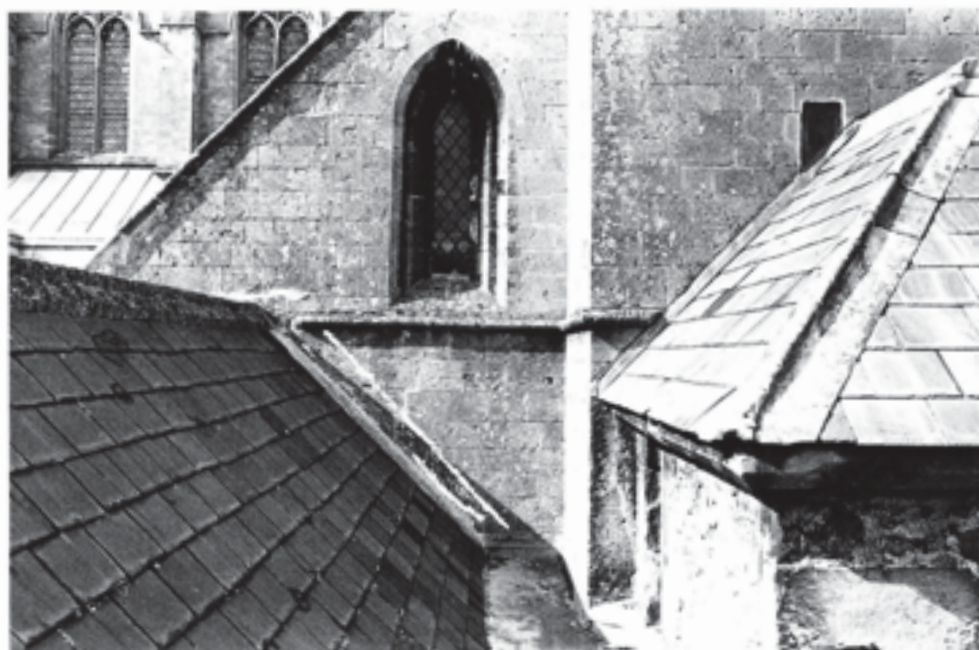
Fig. 298 Detail of the abutment of the present east cloister roof to the west aisle of the south transept. An earlier roof-line is emphasized by the white mortar filling of the flashing chase. The roof of the 1420s stair-turret (Structure 13) is seen on the right, partly blocking an original window to a chamber in the triforium
