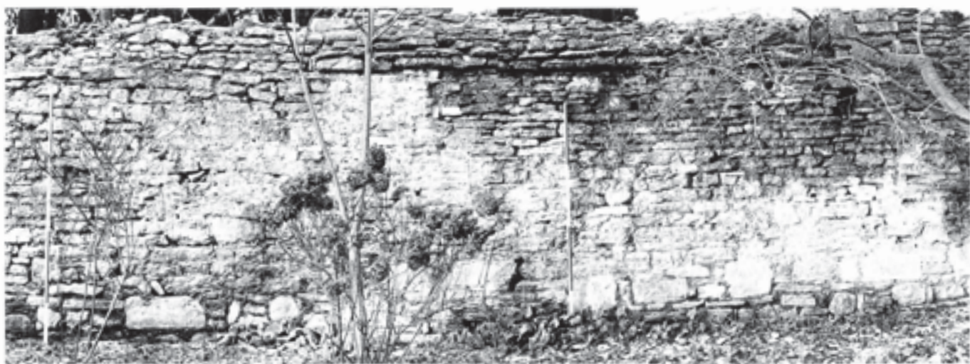
Fig. 362 Camery wall. Remains of the thirteenth-century weathering-course and rubble coping. Viewed from the east, before repair. Scales of 2 m
