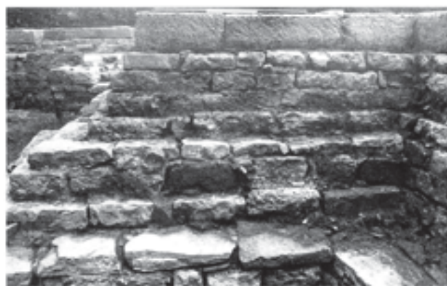
Fig. 201 Stillington's chapel. Stepped buttress foundation (F337b) on the north side of the nave, showing the footing-course of Chilcote stone; west face. Scale of 75 cm
