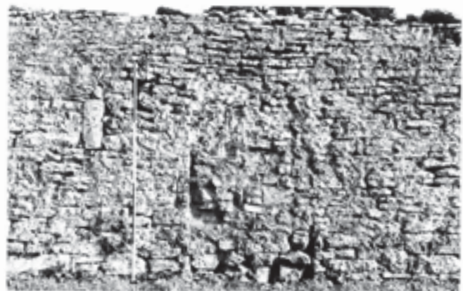
Fig. 364 Camery wall. West face of blocked doorway 'B', and jamb of window 'F' to the left. Scale of 2 m
