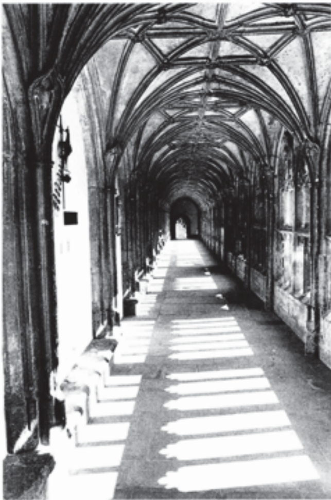
Fig. 263 The east cloister walk, looking south, in 1980, prior to the traceried screen being glazed
