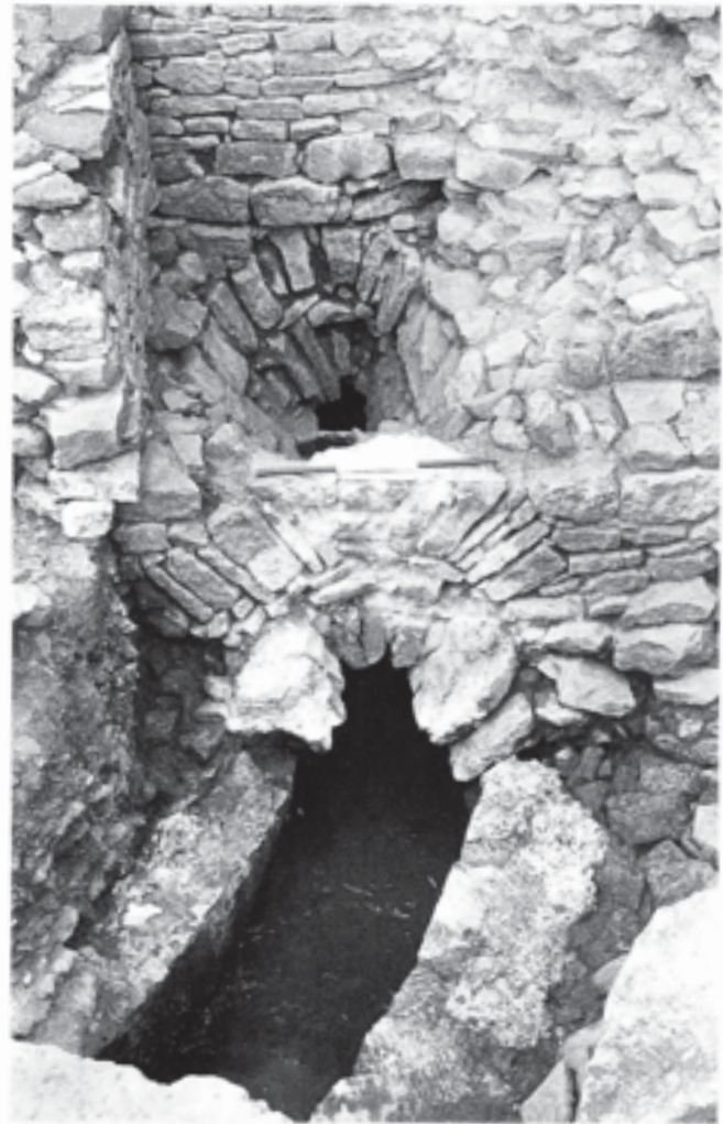
Fig. 393 Junction of Stillington's conduit (seen here with the cover-stones removed) with the earlier medieval vaulted conduit, where it passes under the east cloister. Note the double ring of voussoirs, and the post-medieval hole broken through the vault (behind the 75 cm scale)
