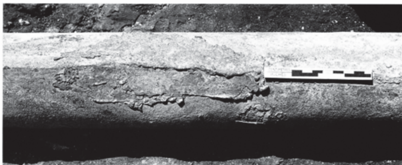
Fig. 428 Example of a soldered repair to the seamed top edge of the lead water-pipe (pipe length 2). Scale of centimetres and inches
