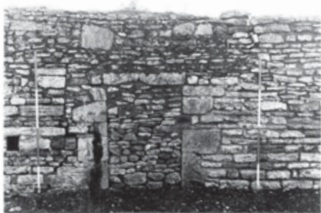
Fig. 359 Features in the Camery wall. A (upper) East face of blocked doorway 'A', before repointing; B (lower) West face of the same feature, during repointing. Note also the open putlog hole on the left. Scales of 2 m (Jerry Sampson)
