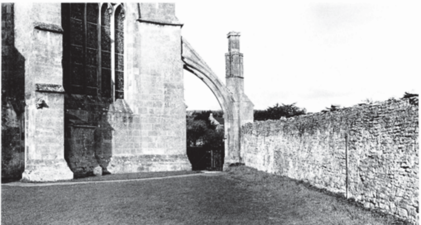
Fig. 367 The north-eastern corner of the Camery, and the buttress-arch adjoining the eastern Lady Chapel. Scales of 2 m
