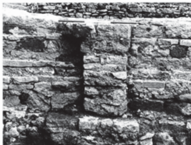
Fig. 211 Pillar-like projection in the foundation of the north wall of Stillington's nave, intended to receive the base of the wall-shaft between the second and third bays. Scale of 75 cm
