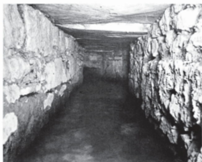
Fig. 403 View west inside Bekynton's conduit (water filled), towards the junction ('K') with Stillington's diversion. Note the reduced aperture to the latter
