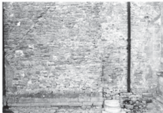
Fig. 150 Outer face of the east cloister wall, showing the abutment scars of the south aisle of the Lady Chapel. Far left is one jamb of the small, infilled doorway that led from the cloister into the Camery; far right is one jamb of the infilled doorway into the nave of the Lady Chapel. Scale of 2 m
