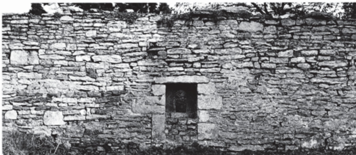
Fig. 366 Camery wall. West face, after clearance, showing the fifteenth-century window-recess 'C', with masonry blocking in the lower part (cf. Fig. 396)
