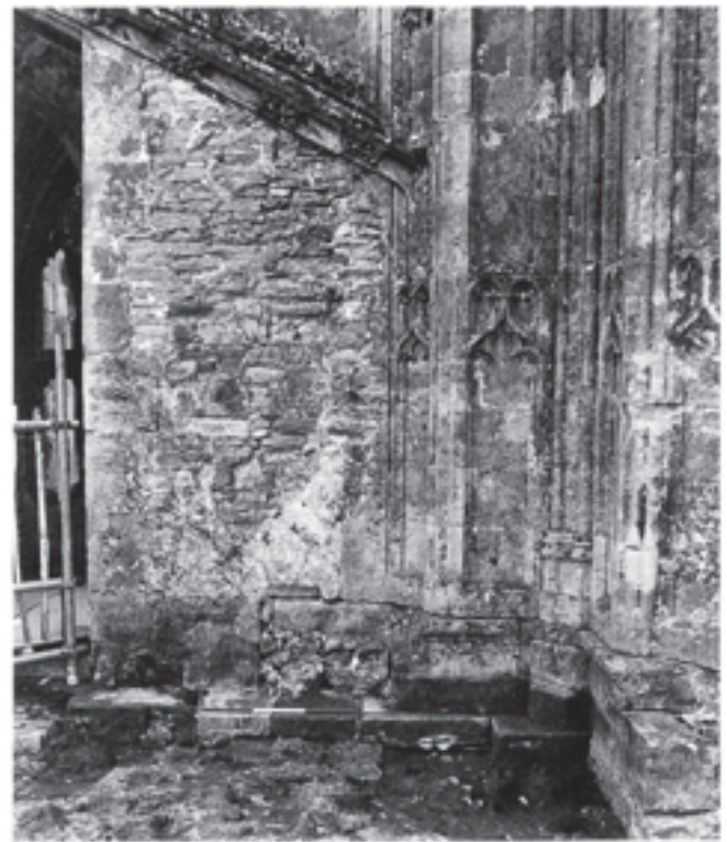
Fig. 239 The north-west corner of Stillington's nave. The 75 cm scale rests on the remaining original Douling stone paving, upon which there was formerly a wall-bench
