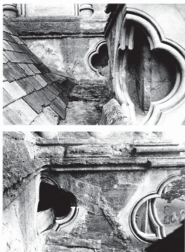
Fig. 287 South-west tower. Quatrefoil niches and hacked-off gablets, above the west cloister roof. A (upper) South face of tower, with south-east buttress on the right; B (lower) West face of the south-east buttress
