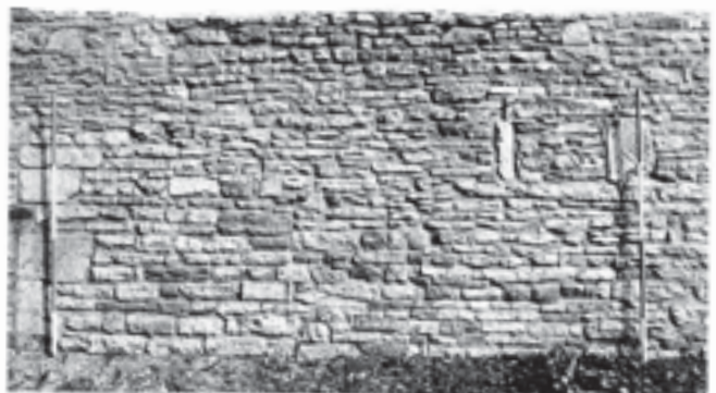
Fig. 365 Camery wall. West face of window 'E', after repointing. The jamb of doorway 'A' is visible on the far left. Scales of 2 m (Jerry Sampson)
