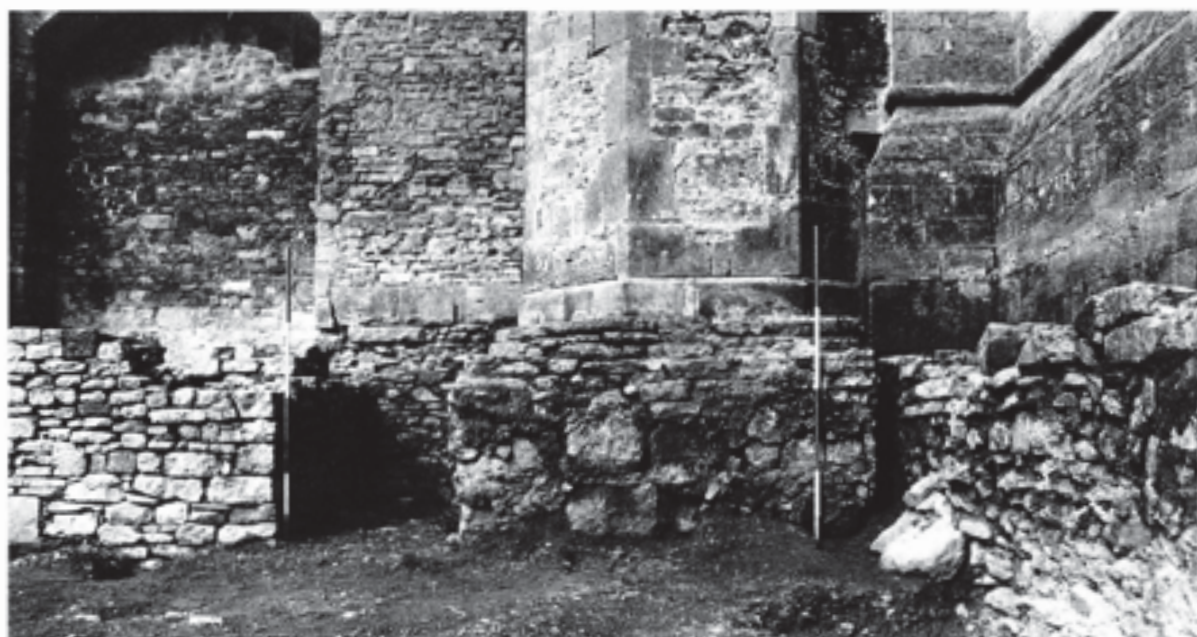
Fig. 313 Different foundation characters revealed in the north-west corner of the Camery. Right small broken rubble and mortar filling the foundation trench of the south transept, c. 1180. Centre large boulders and ample mortar forming the foundation raft of the library stair-turret, c. 1425. Left coursed rubble of the Holy Cross chapel, c. 1495. Scales of 2 m
