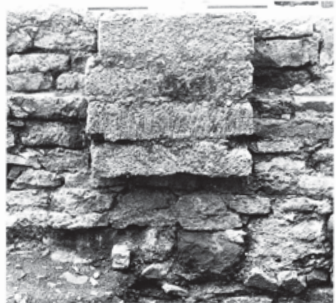
Fig. 207 Stillington's chapel. Corbelled foundation of Chilcote blocks for the support of a wall-shaft between the first and second bays on the south side of the nave. Scale of 75 cm
