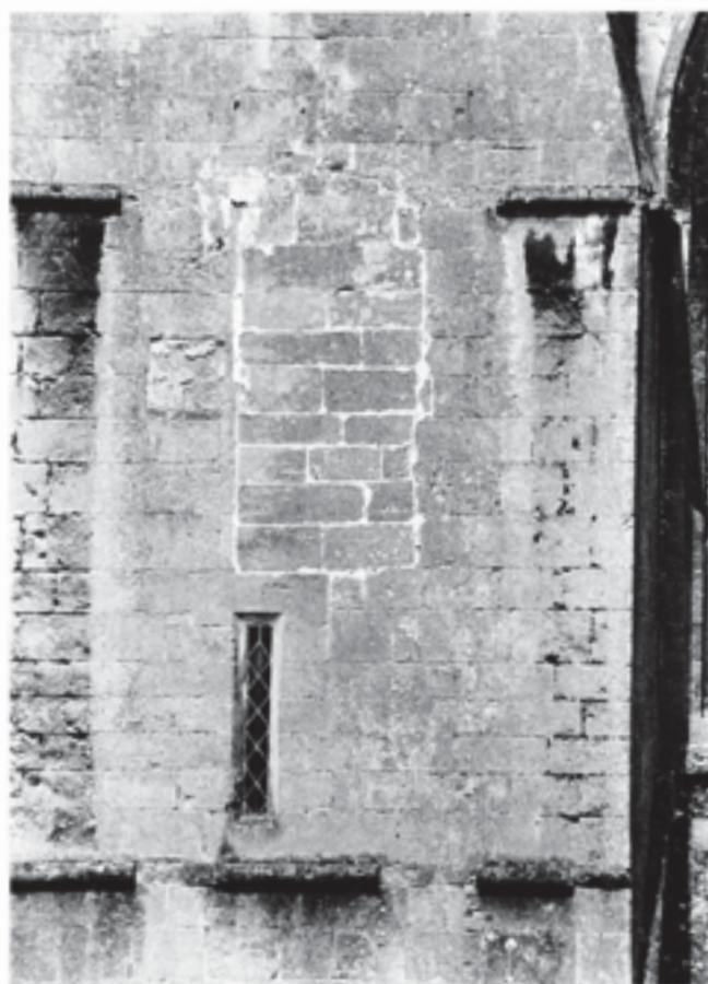
Fig. 231 Blocked high-level doorway and scars left by the removal of the linking bridge between Stillington's chapel and the south transept of the cathedral
