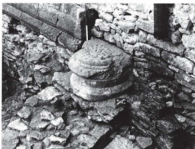
Fig. 140 Lady Chapel. The west respond-base of the arch between the nave and south-west chapel, looking south-west. A single piece of lias paving can be seen on the chapel-side (left of the base), and a fragment of medieval tile paving ( fleur-de-lys ) on the nave-side (Fig. 137, area H). Scale with 25 cm divisions
