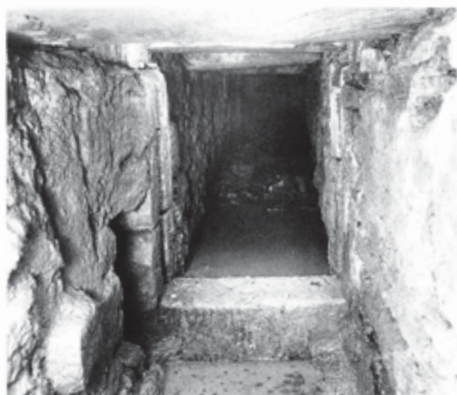
Fig. 402 View west inside Bekynton's conduit, showing the original sluice ('H') and bar forming a step in the floor. The opening to a small culvert (F936), heading south towards the millstream, can be seen on the left
