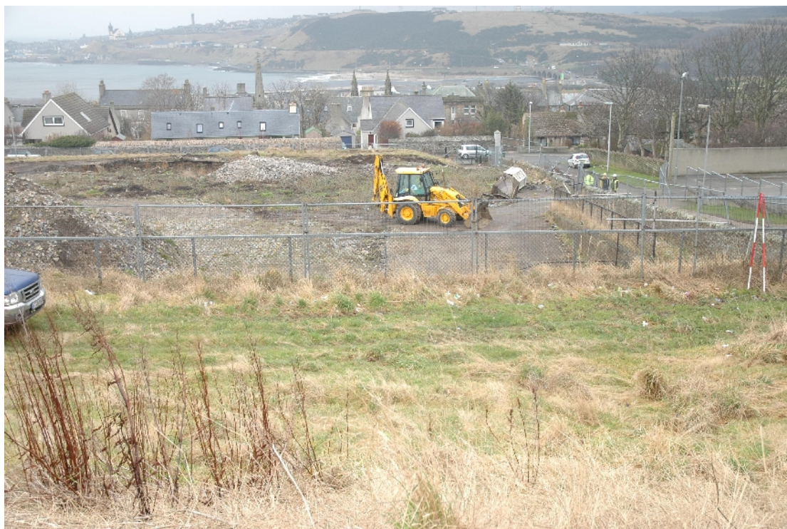
Illus 1 Looking E across the site towards Walker Avenue. Photograph taken from terrace Area D, looking across Areas F and A.
