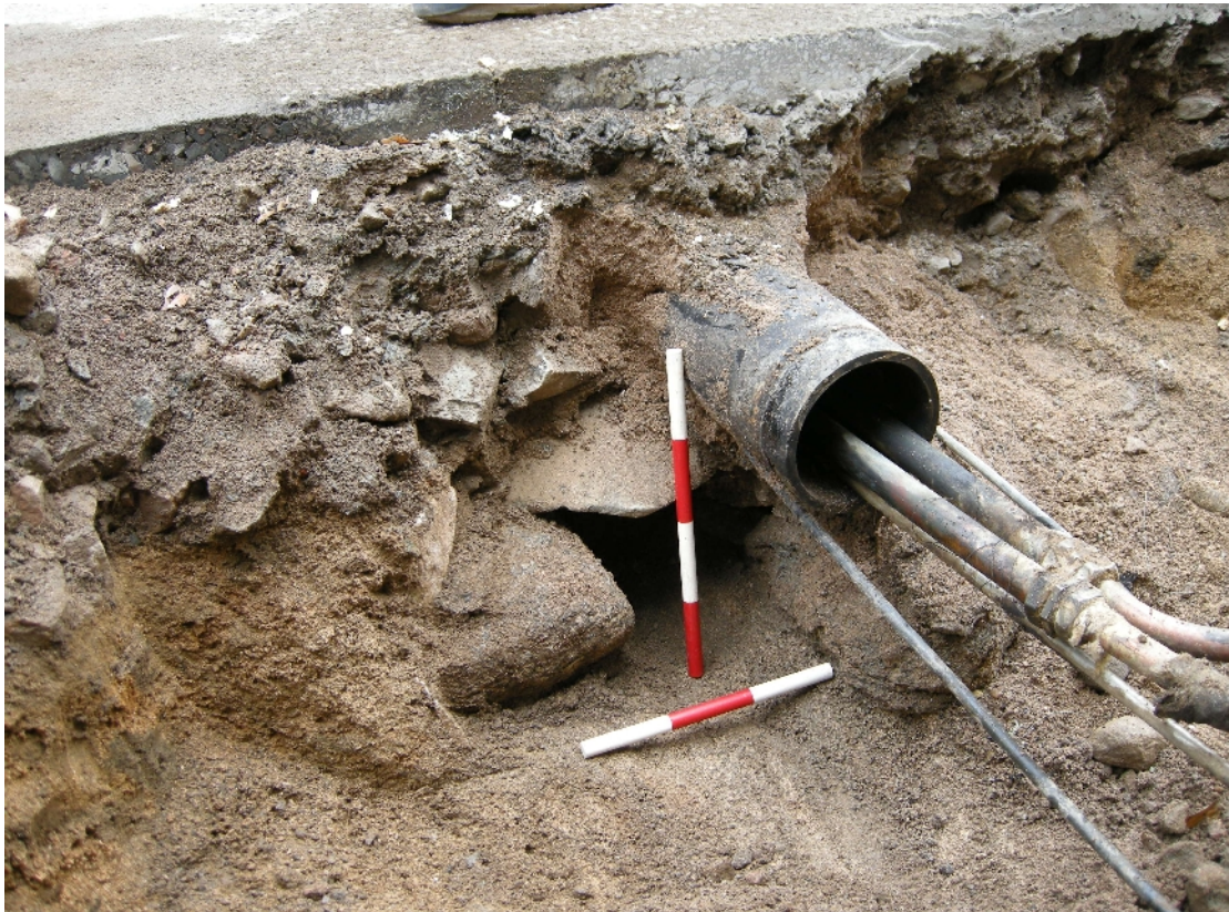
Illus 3 Trench 1. Section of stone drain shown below duct for service pipes
