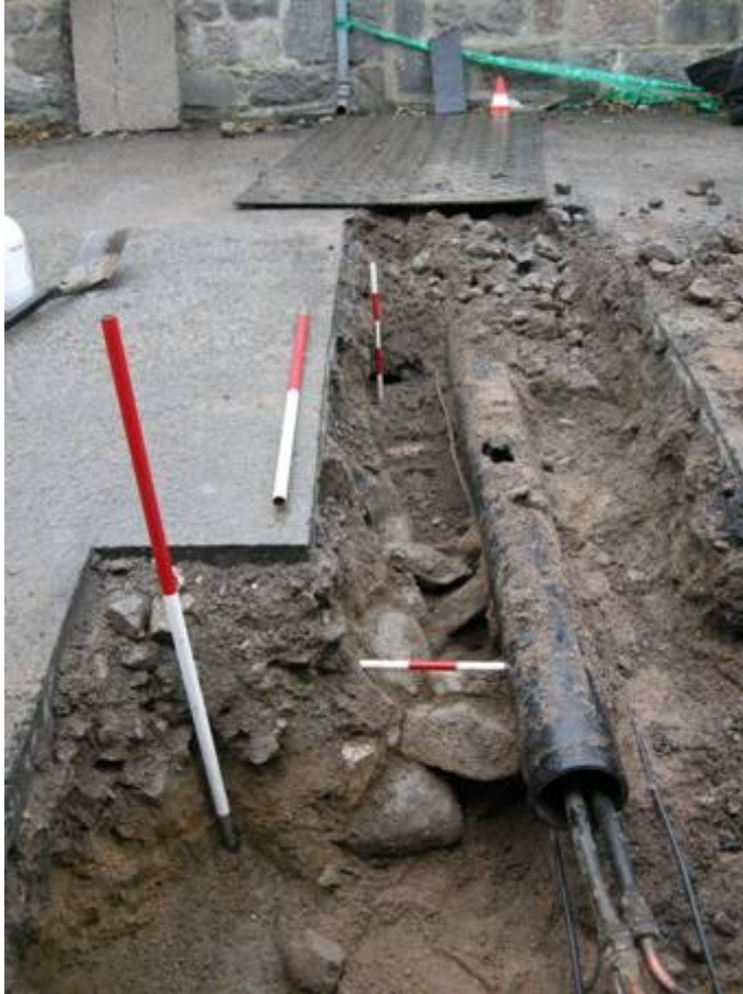
Illus 4 Looking W along trench 1, showing stone drain on LHS of pipe duct
