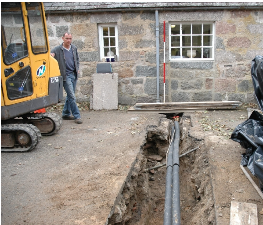
Illus 5 Looking W along trench 1, showing new service pipes and the stone drain (LHS) in relation to doorway (now window) in W building.
