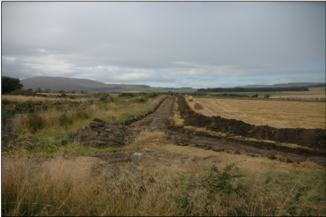
Illus. 5: Cable trench corridor, looking S from N side of farm buildings.
