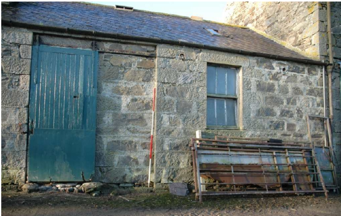
Illus 9 Detail of N end of stable block showing recessed sliding door D11 and window W9
