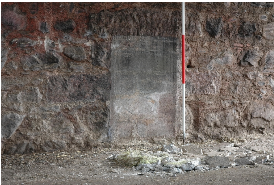
Illus 12 N wall of S range, Detail of W4, showing walkway has blocked base of wall, making window appear low.
