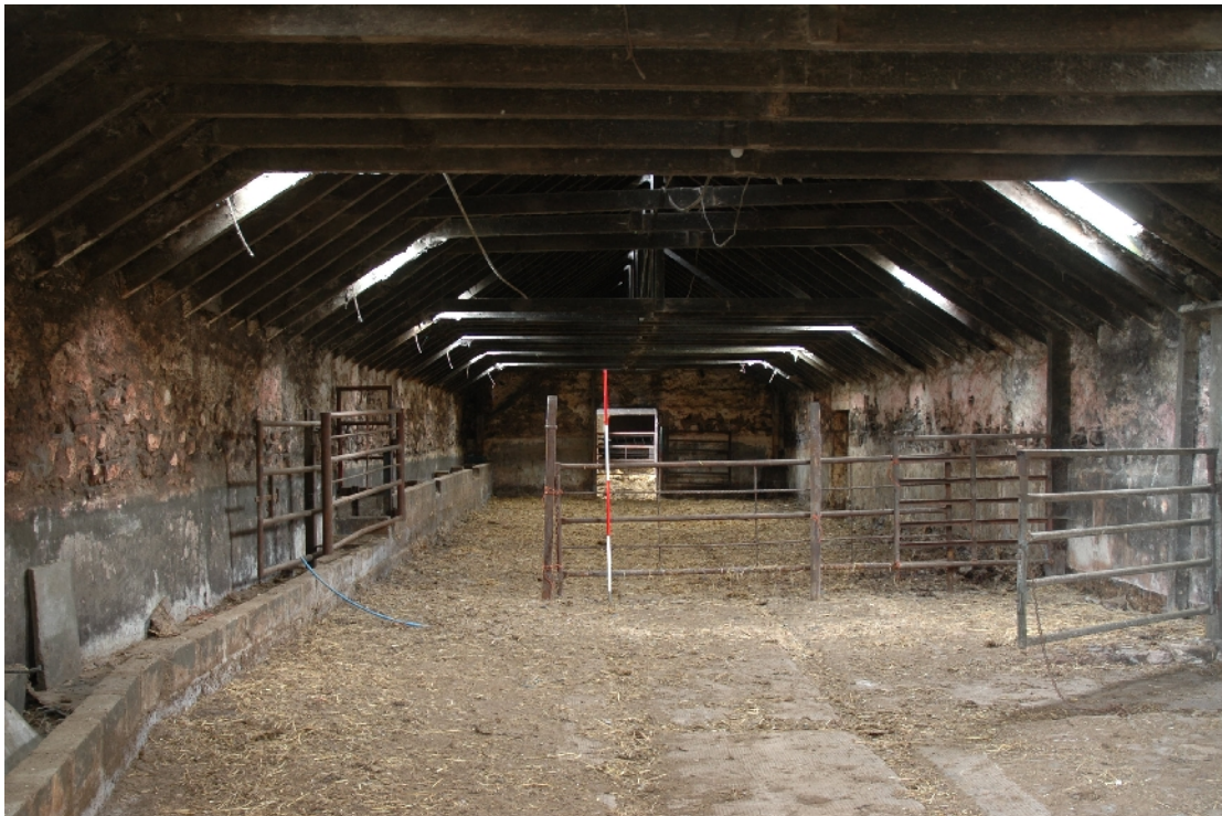
Illus 17 Interior of E range central concrete drain and original cobbles just visible.
