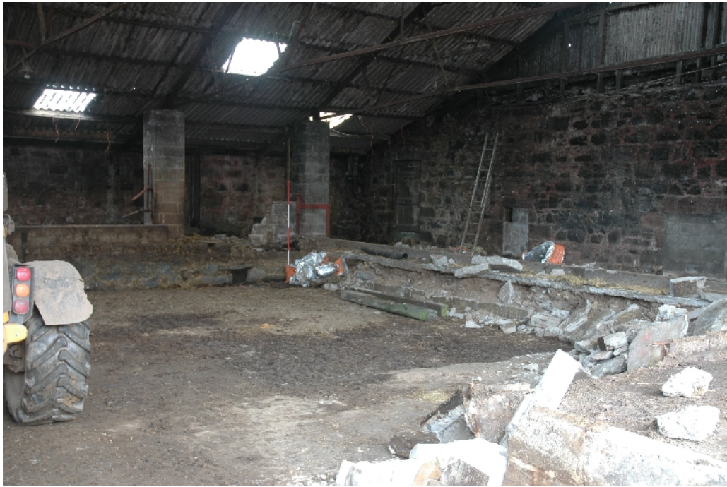
Illus 11 N wall of S range, looking SE across central court. W2 visible beside ladder
