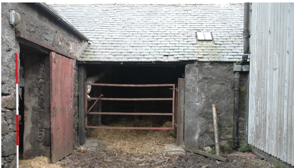
Illus 23 Roof of later 19 th century range of buildings abutting S range
