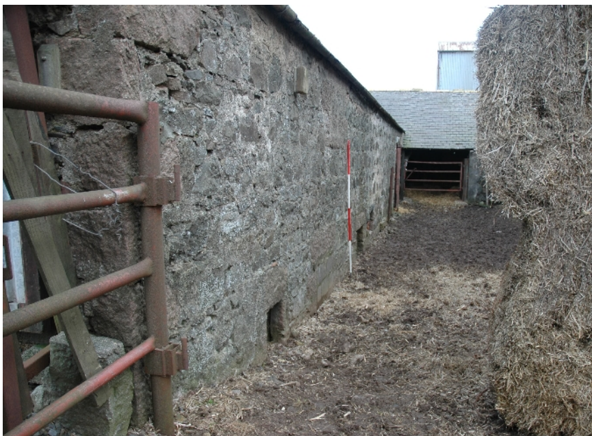
Illus 13 Oblique view looking E along S wall of S range. W5 in foreground
