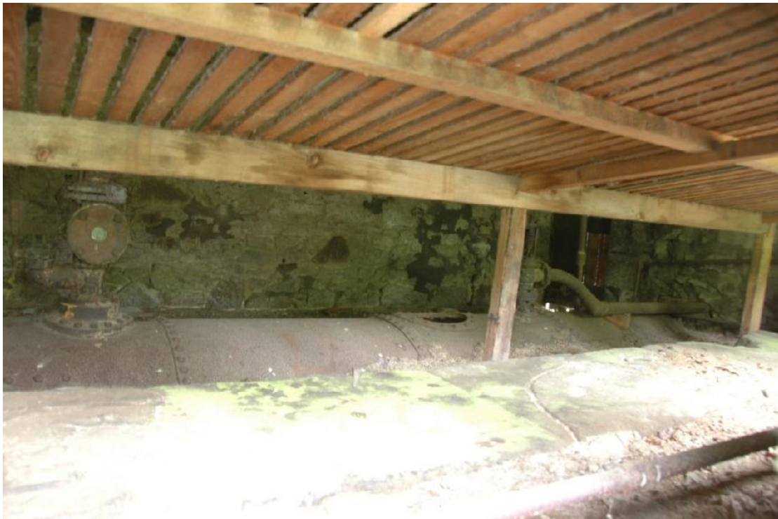
Illus 14 Horizontal boiler running full length of Building 1 1 st floor. Seen through window W9 The brick- built flue and ash pit in the S wall of Building 1 indicate a secondary break-through, as do the smaller break-throughs for the iron steam pipes. This would indicate that Building 1 (W end) may have pre-dated the use of steam power and been adapted in the mid-19 th century. The SW corner of the chimney abuts Building 1 W
