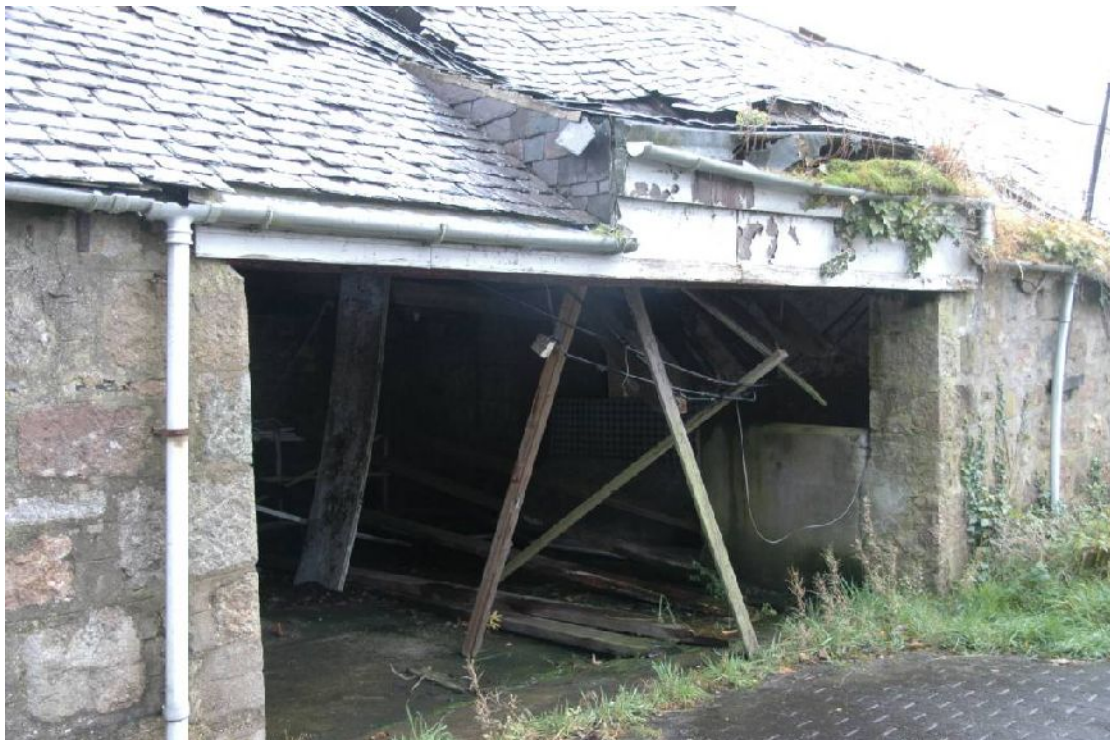
Illus 6 E wall door D2 showing the higher roof over original cart door.
