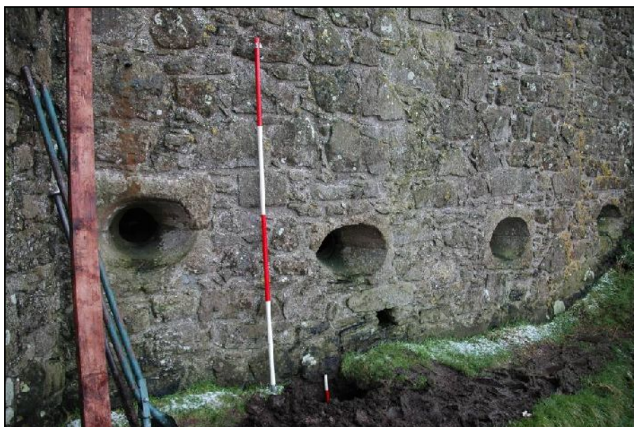
Illus 7: Position of posthole to the left of the central gun loop
