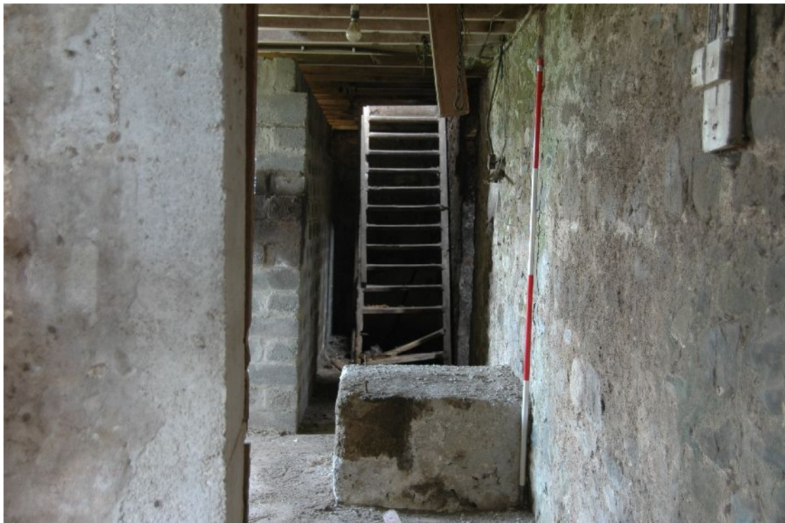
Illus 4 Looking N in Area B. Bruiser base with hopper above. Stair to loft behind.
