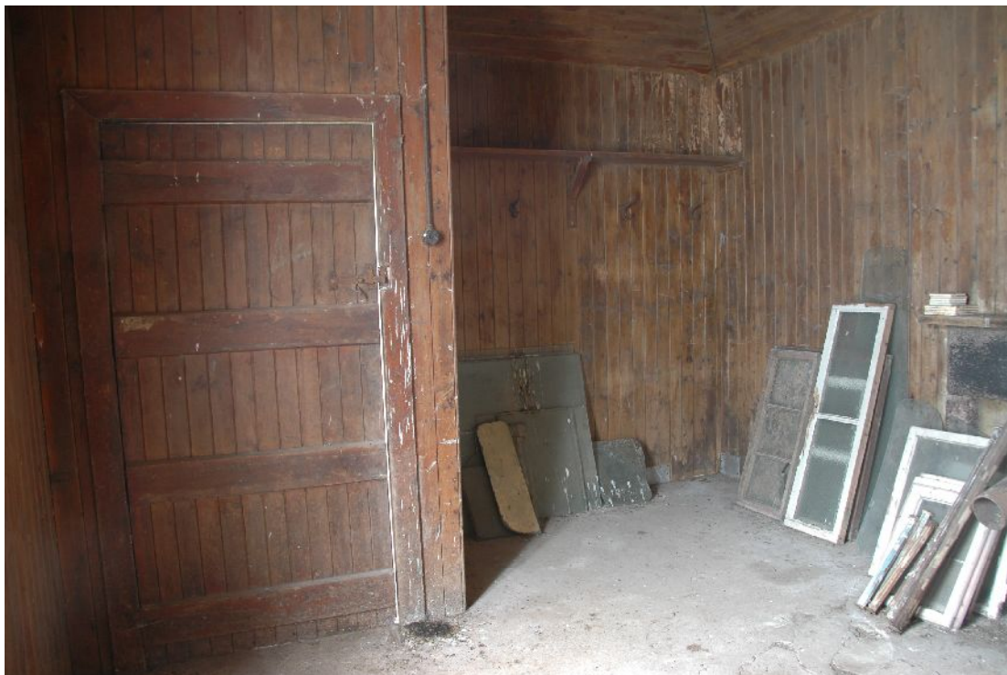
Illus 9 Bothy internal view looking NW into bed alcove. Fireplace visible behind stacked windows on RHS
