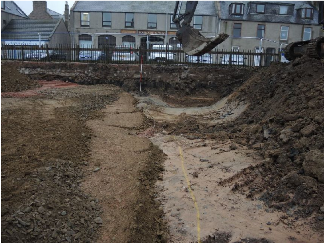
Illus 9 NE sector showing clean hardcore put in to new building level
