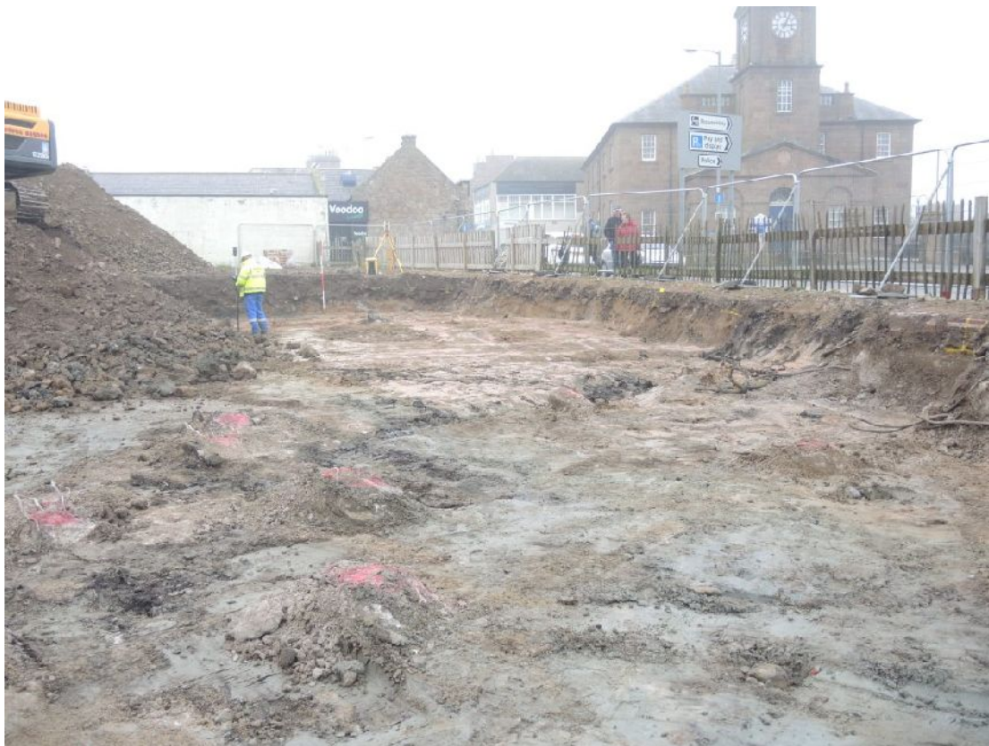
Illus 7 W sector general. Red marks indicate concrete foundations in natural clay
