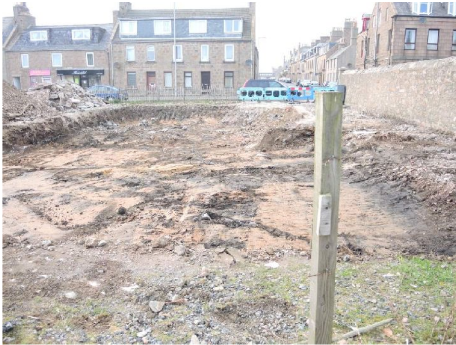
Illus 5 NE sector. Post-demolition fill removed to natural clay. Piles from flats visible
