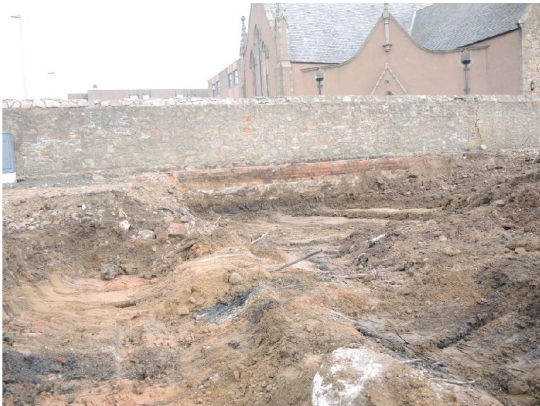
Illus 6 NE sector. Piles and concrete ring beam from 20 th C flats
