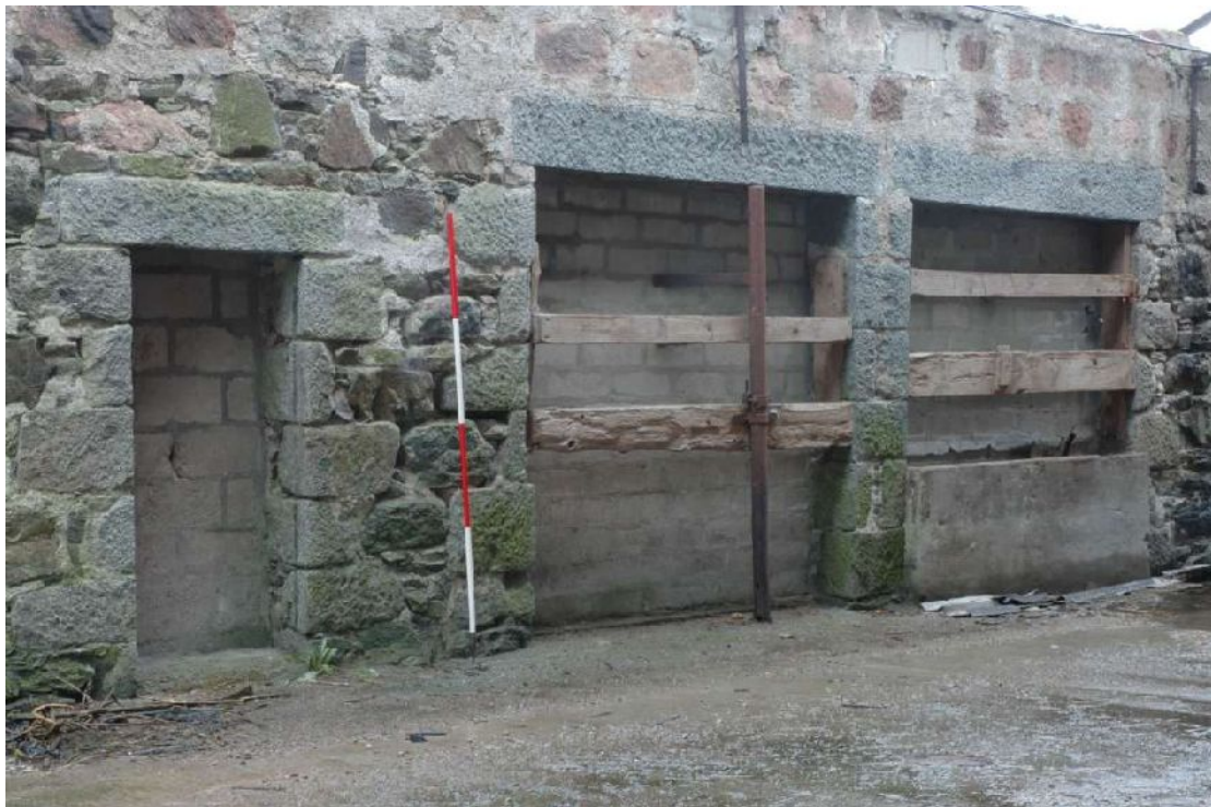
Illus 7 N wall of S range. Detail of D2 and cart bays D3 and D4
