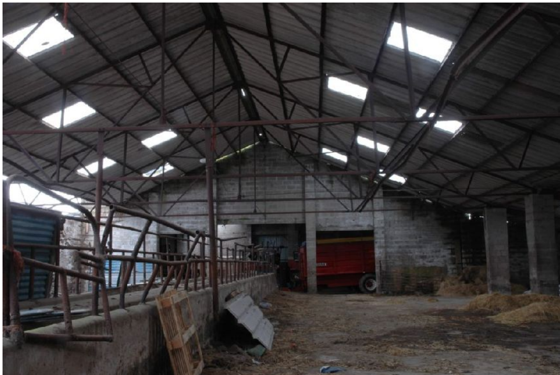
Illus 8 Looking W along Building D with central feed pass on LHS
