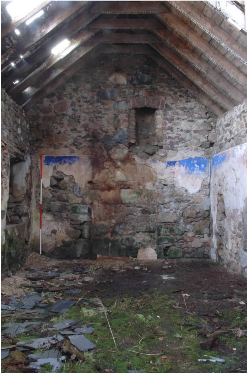
Illus 17 4A. Interior view of E wall with blocked ground level fireplace and brick fireplace at attic level
