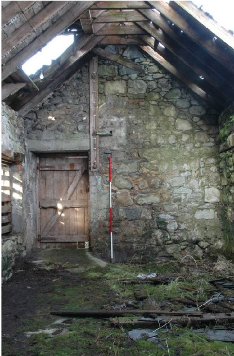
Illus 18 4A internal view of W wall showing blocked fireplace at attic level. Note at RHS the original, lower roof pitch.
