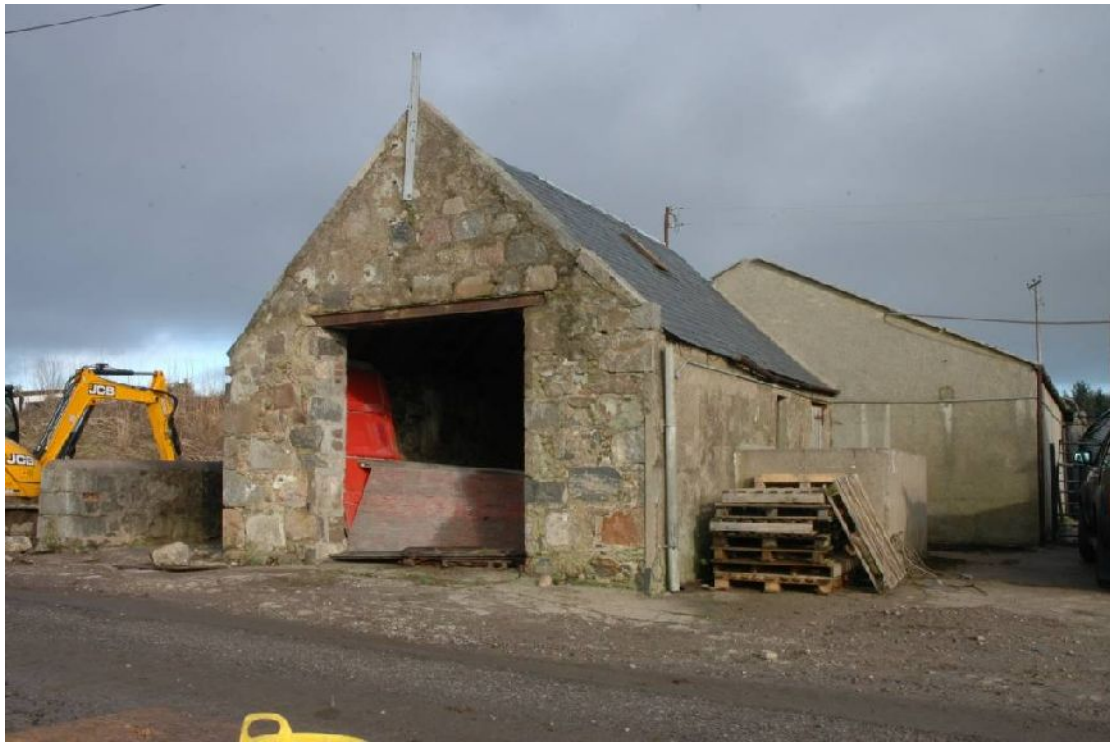
Illus 7 B2 S wall of 2A – part of 19 th century W range.
