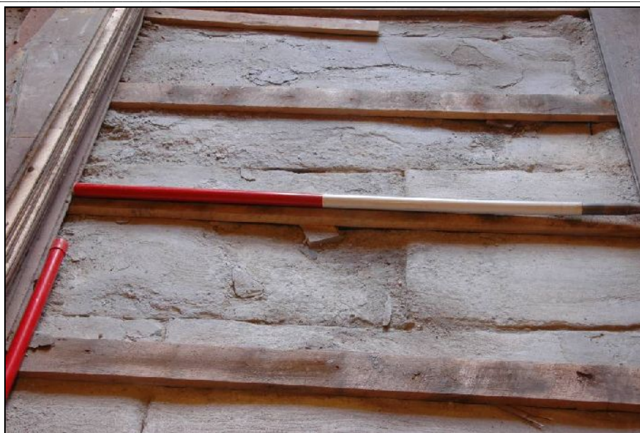
Illus 5: Detail of flagstones below the wooden flooring. Note the wedge below the batten in the centre.
