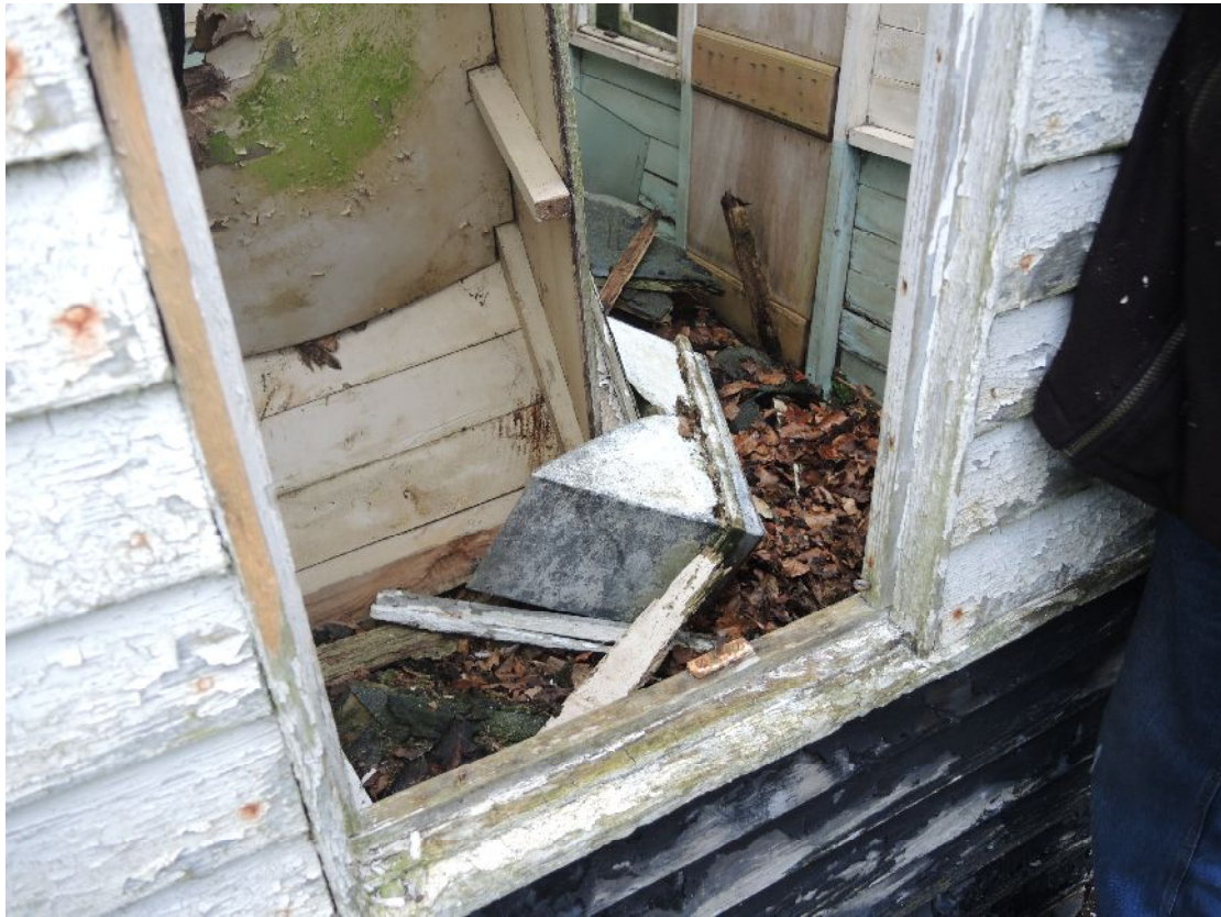
Illus 9 Chimney visible in debris on floor 2014
