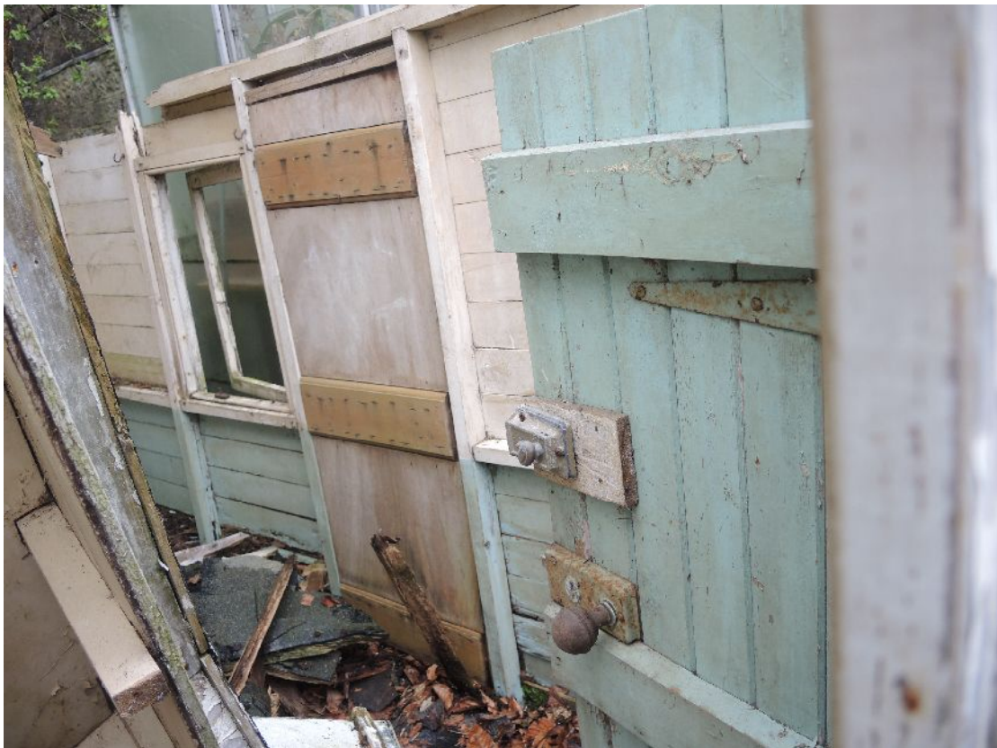
Illus 8 Internal view of N wall 2014. Open door D1 in foreground. Dummy door D2 and W3 in background
