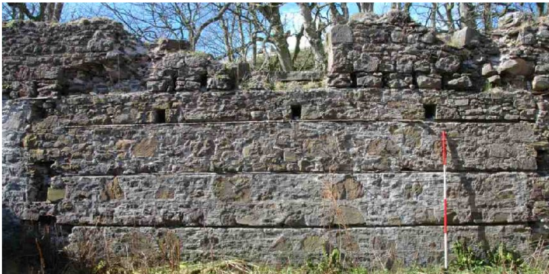
Illus 4 Detail of inside of W wall in central 'room' showing fixings for timber lining and ventilation holes D-F. The raggles of the former internal partitions can be seen on either side of the picture.
