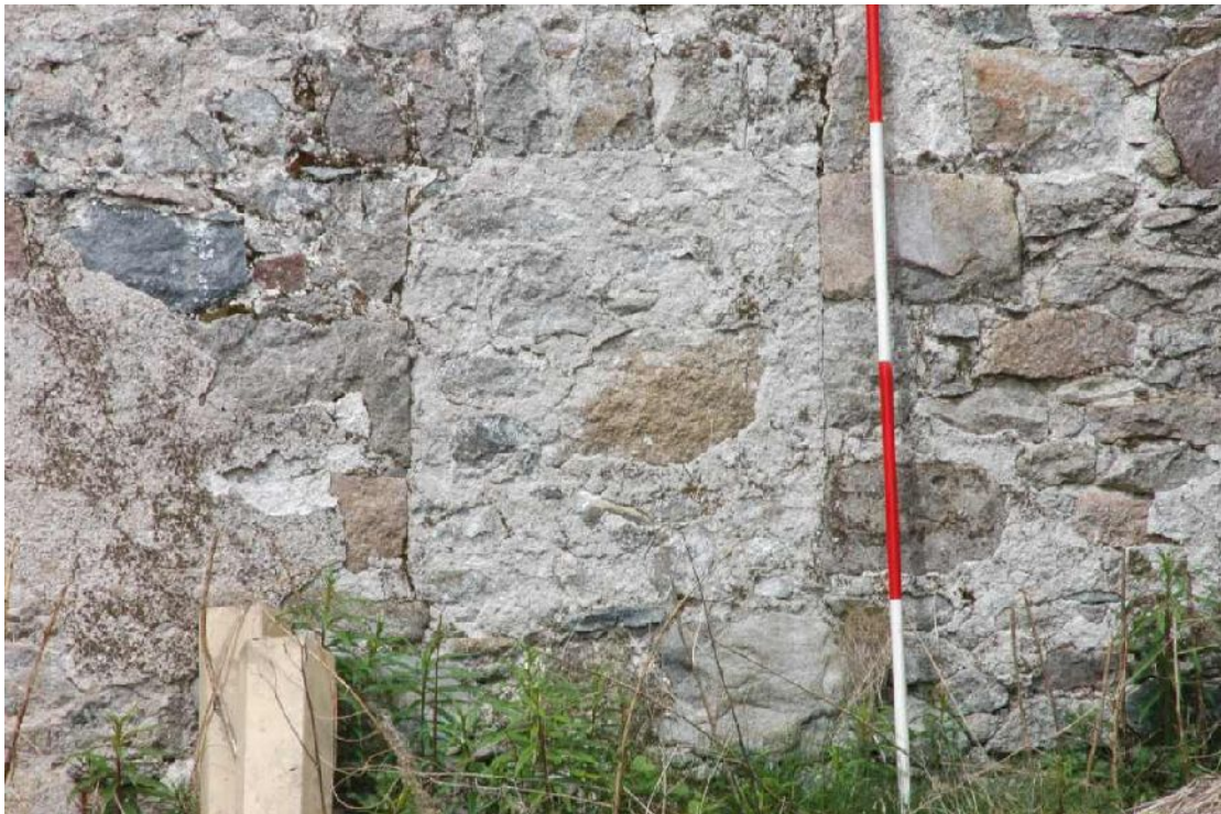
Illus 10 detail of blocked window in S wall of N Range, East Court
