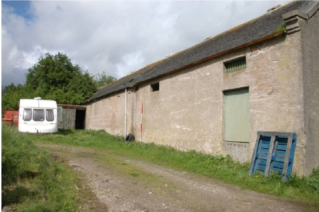
Illus 13 W wall of W range of West Court from outside, looking N. Ranging rod indicates the probable position of the wall between the bothy with loft above at S end and the stalls with vents at N end.
