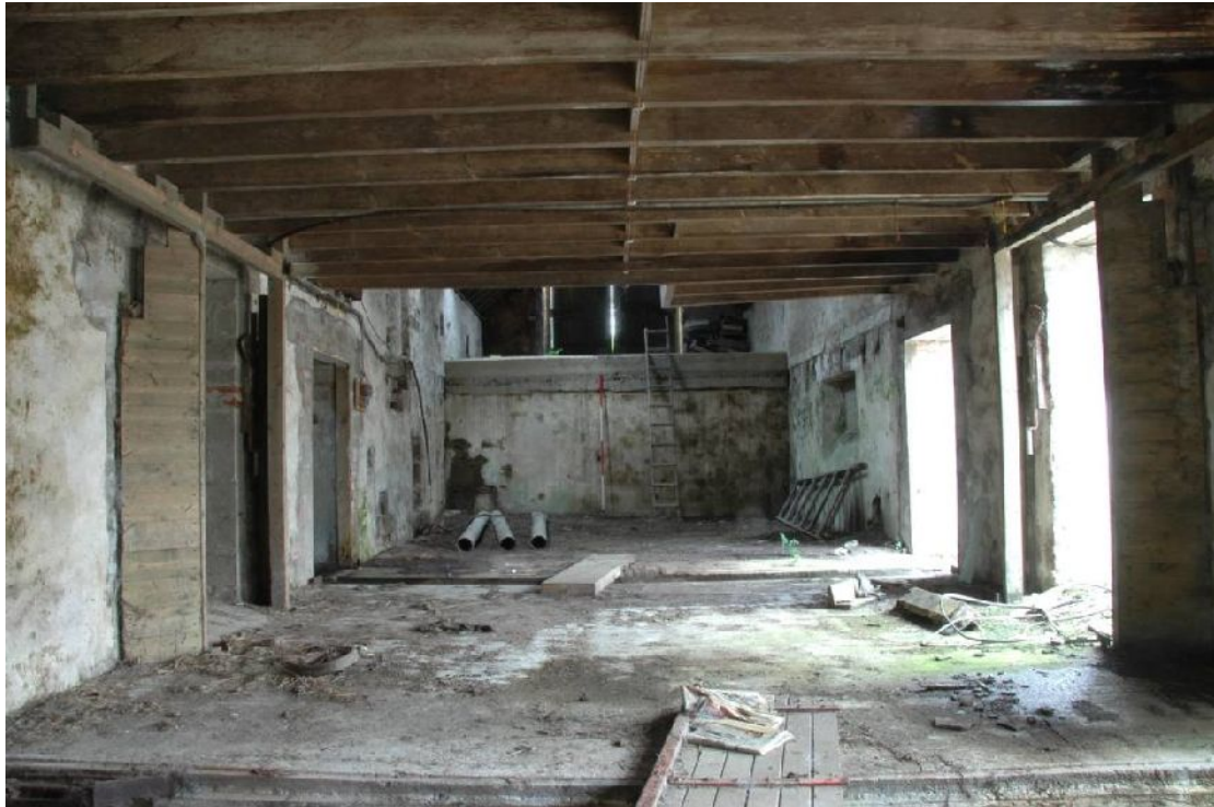
Illus 19 Interior of mill from below loft of East Court, W range (by D7)
