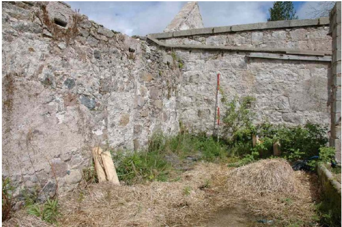
Illus 5 Stonework in NW corner between N and E ranges of East Court
