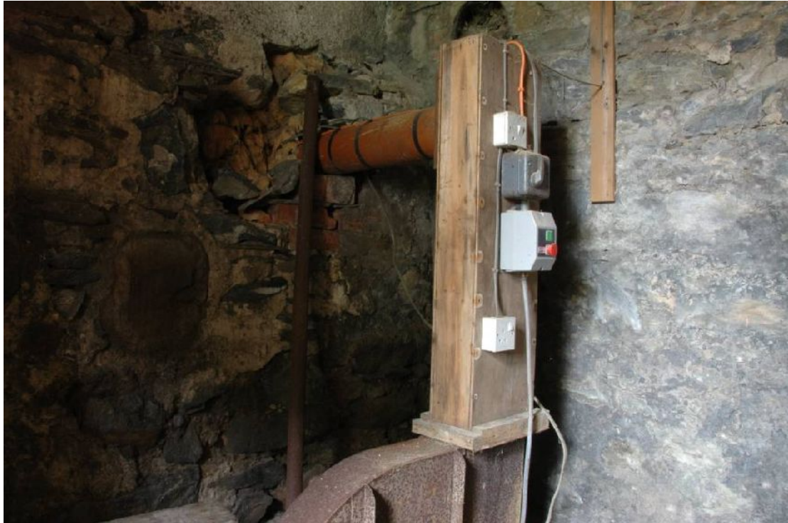
Illus 24 Drive for organ bellows with vent through pipe in wall. Note earlier blocked openings for heating.
