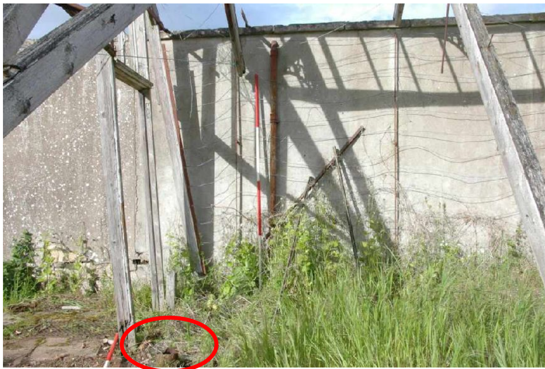
Illus 21 NW end. Large cast iron pipe in foreground marked by red circle, smaller diameter pipe up wall beside ranging rod
