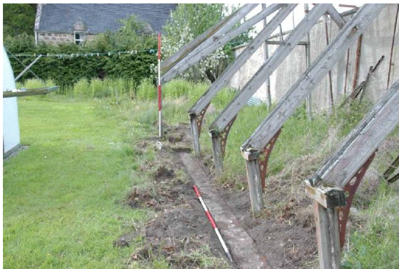
Illus 7 Looking N along side wall showing brick foundation and displaced wall timbers
