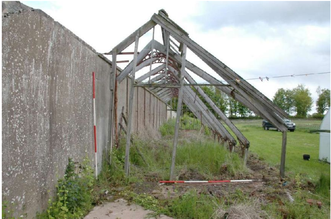
Illus 11 NW gable showing displaced door jambs.
