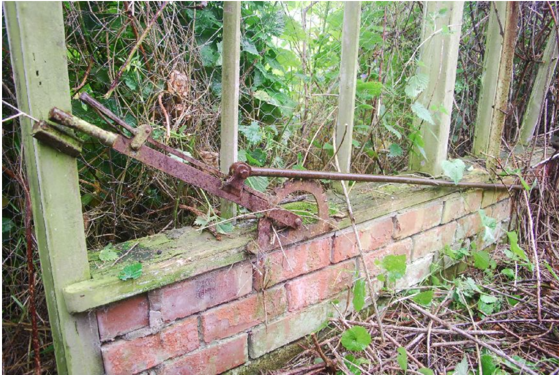
Illus 25 S gable in 2009, showing ratchet mechanism for opening the lowest (vertical) windows. This mechanism was removed and is now in use at Pitmedden, Aberdeenshire. (Photograph R Grant).
