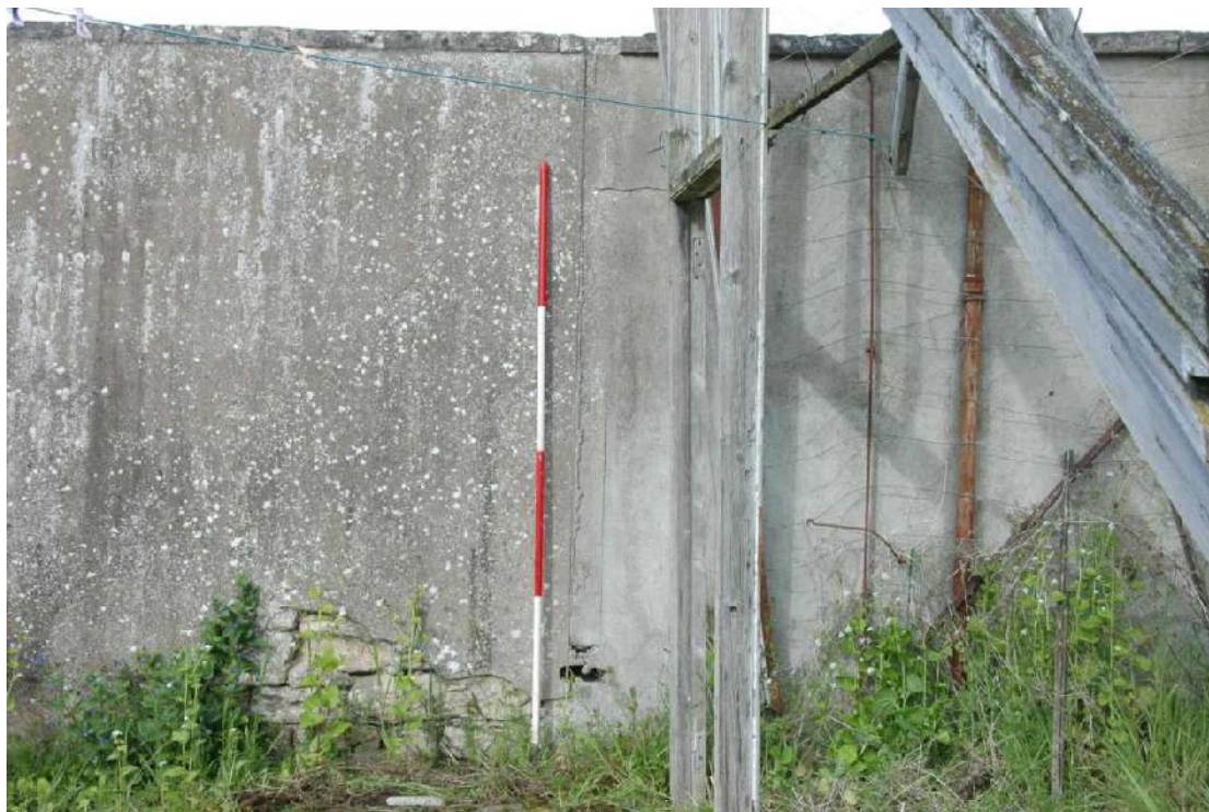
Illus 5 NW gable, looking E to the garden wall. The raggle of the original wall line of the glasshouse is visible to the RHS of the ranging rod, with an angled slot in the wall face where the wall plate of the gable wall would have been set.
