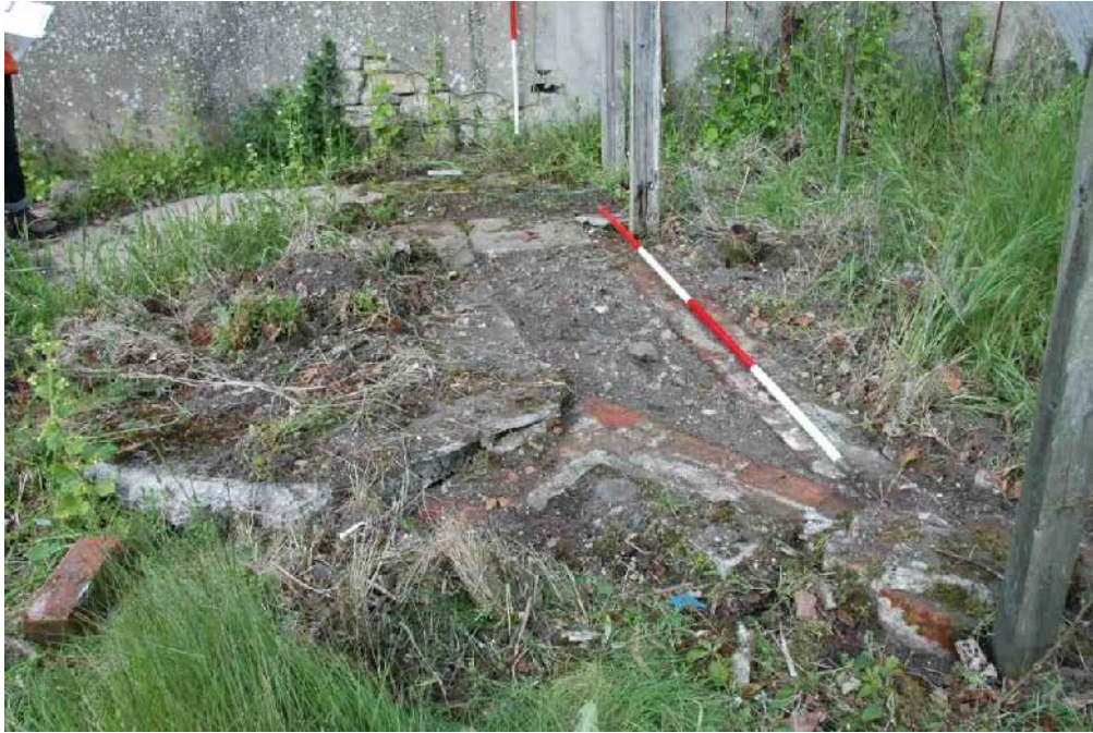
Illus 6 NW end, looking E, showing the line of the original wall foundation (below horizontal ranging rod). The raggle of the original wall and the slot for the wall plate can be seen in the garden wall to the RHS of the vertical ranging rod. The displaced door jambs can be seen to the RHS of the foundation. To the LHS of the wall foundation can be seen the brick and concrete foundations of a path and other possible structures.
