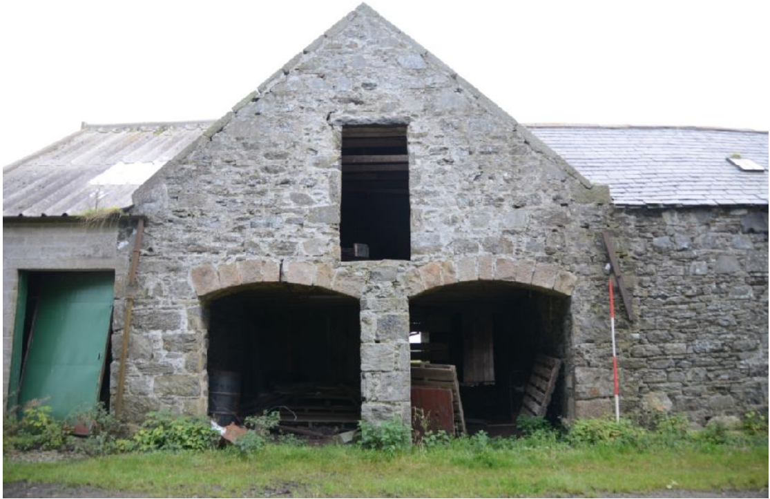
Illus 12 Cart bays in N end of W range with loft door above
