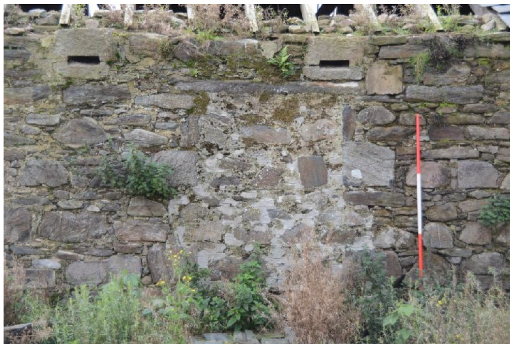
Illus 9 N wall N range. Blocking F5 to LHS of ranging rod. Vents F4 above
