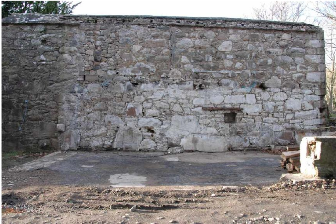
Illus 14 General view of the garden wall and the foundations of the workshop.
