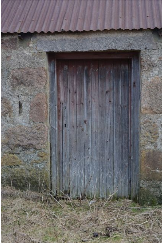
Illus 19 Building 3 D2. showing use of grey granite lintel with quarry marks
