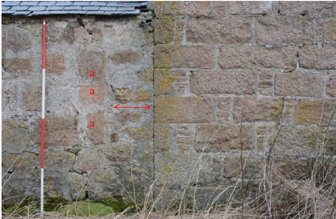
Illus 14 Wall between Building 1 (RHS) and Building 2 (LHS) with infill between (marked by arrows). Three chamfered rybats marked 'a' denote original end or opening in Building 2.
