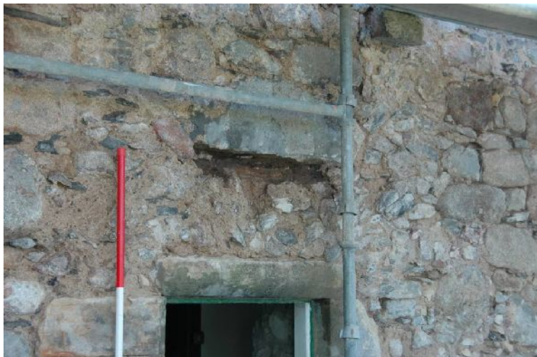
Illus 24 F5 visible top at RHS of scaffolding. Stone above D2 just below horizontal scaffolding
