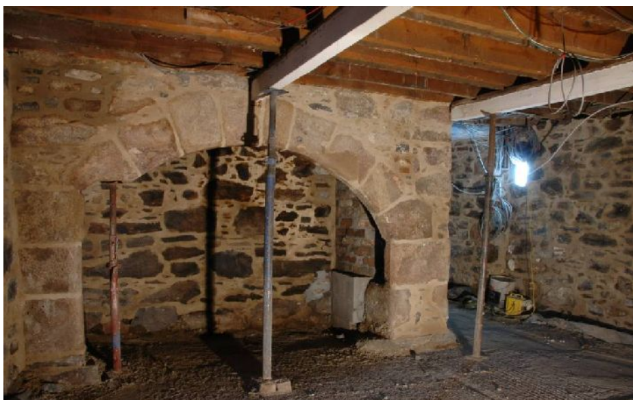
Illus 49 Top and centre, the modern fireplace with 16 th -century fireplace emerging. Bottom, the 16 th -century fireplace. Note the low ceiling cut into top of fireplace
