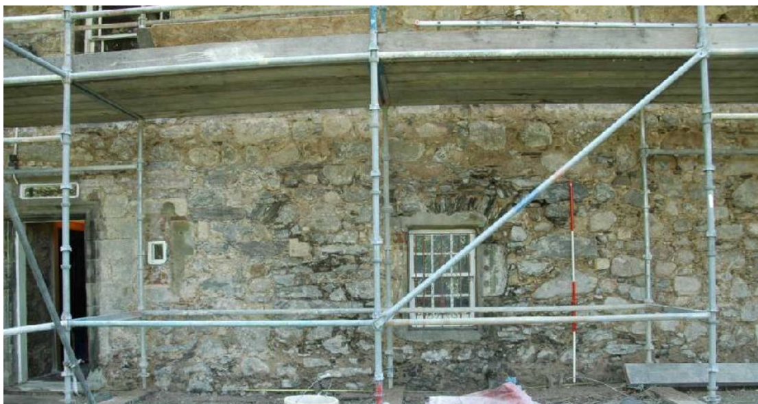
Illus 9 Detail of wall between pend and tower when harling removed. Note the more regular courses begin just below the scaffolding planks
