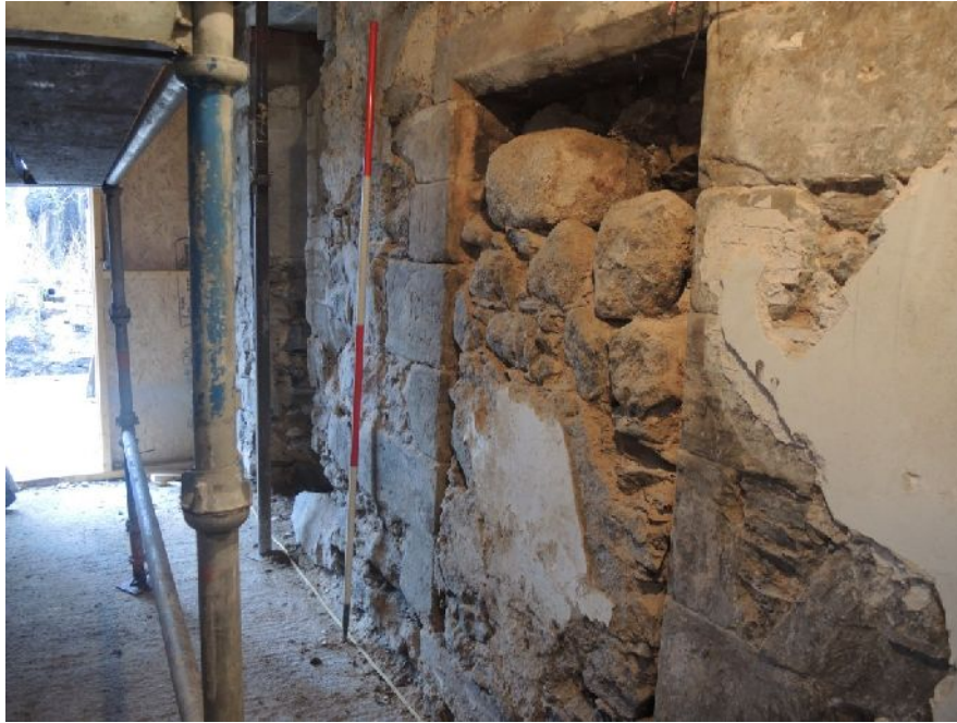
Illus 35 Pend blocked doorway D7 with outer stone blocking and plaster partly removed. Looking towards the garden end of pend.
