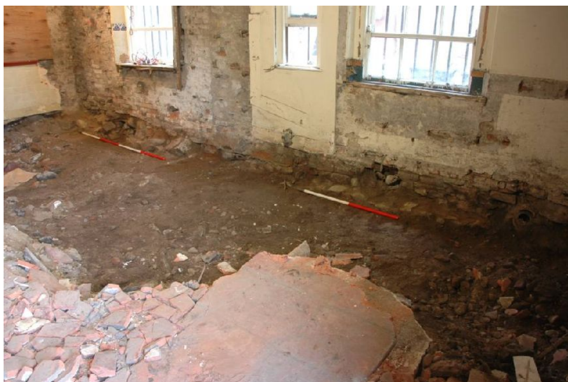
Illus 68 Kitchen. E wall showing the earlier stone wall foundation visible after removal of the internal floor levels.
