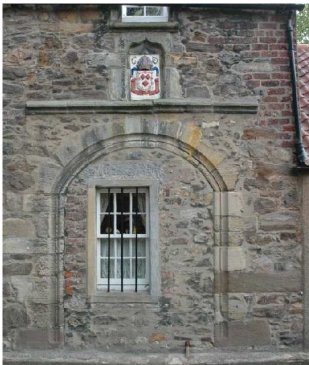
Illus 31 Street pend arch and detail of possible repairs on RHS
