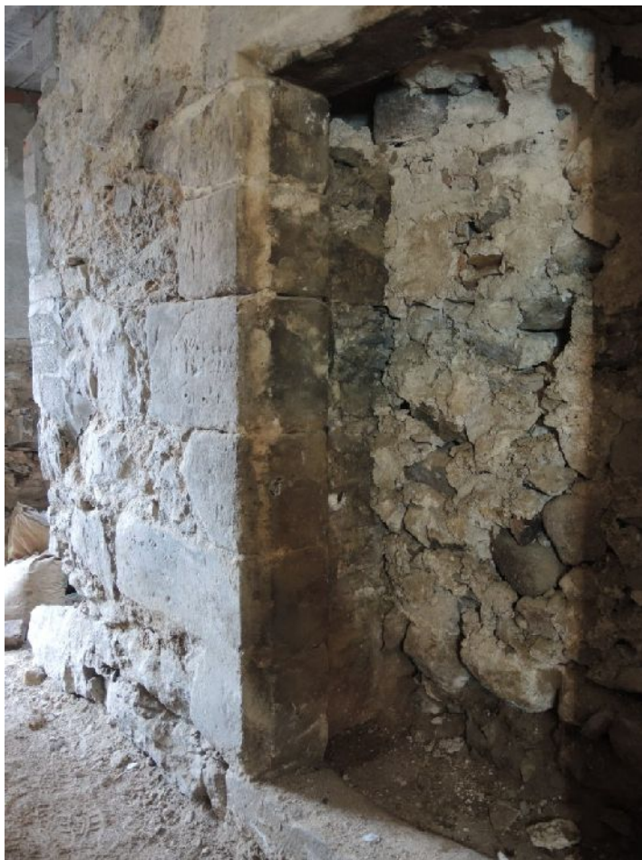
Illus 36 Pend doorway D7 with pend blocking removed, showing rough inner blocking on kitchen side.
