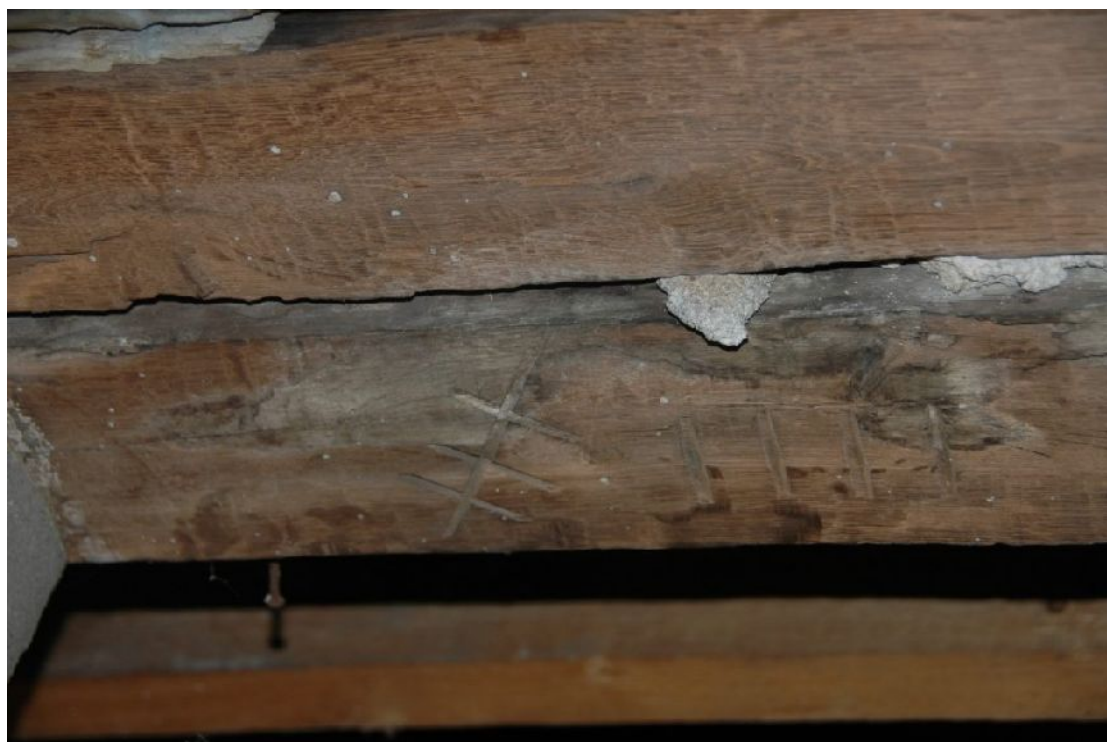
Illus 13 Re-used timbers across hatch through wall of tower into roof space. Carpenter's marks.
