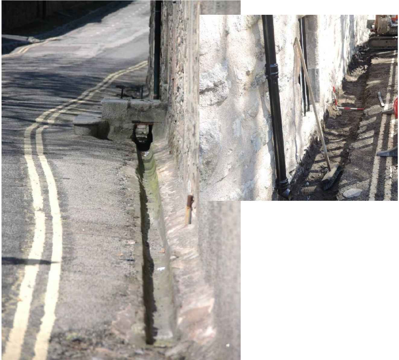
Illus 85 Stone drain along street frontage, before re-instatement (above) and during re-instatement (RHS).
