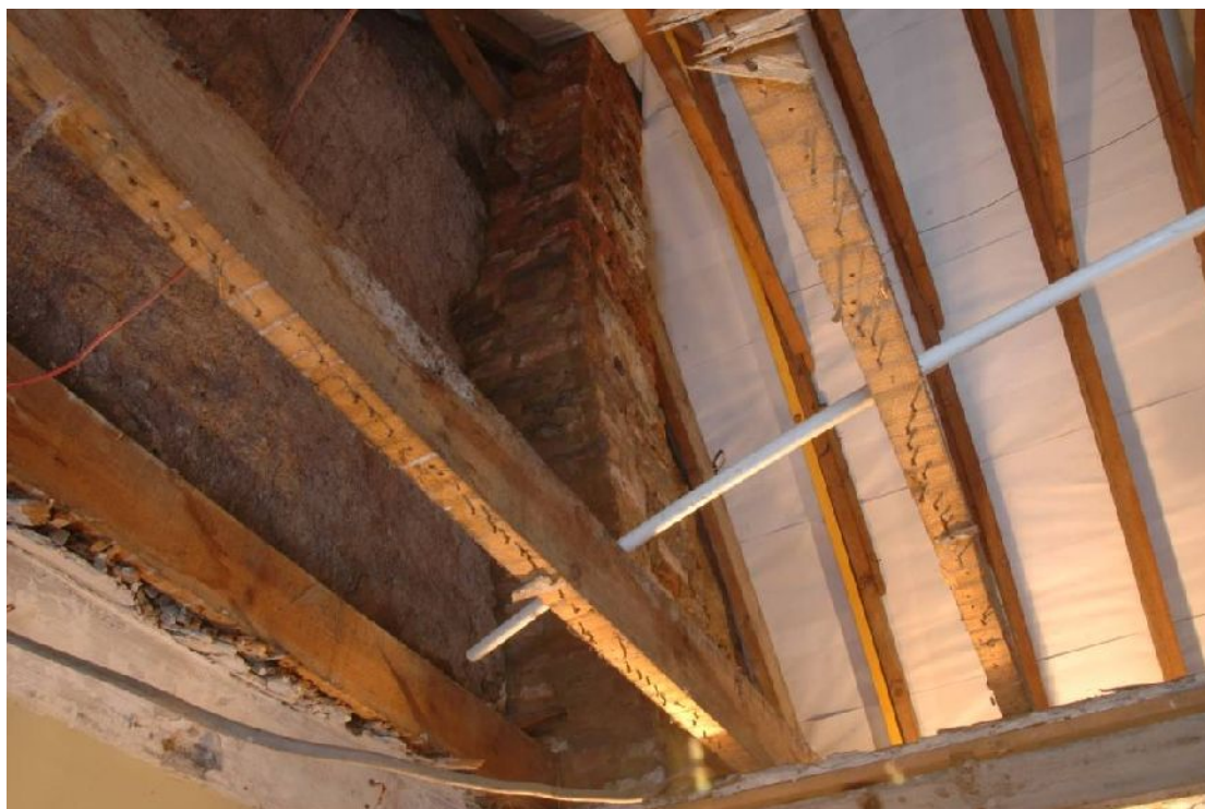
Illus 17 Secondary brick chimney at N end of kitchen, abutting outer wall of pend.
