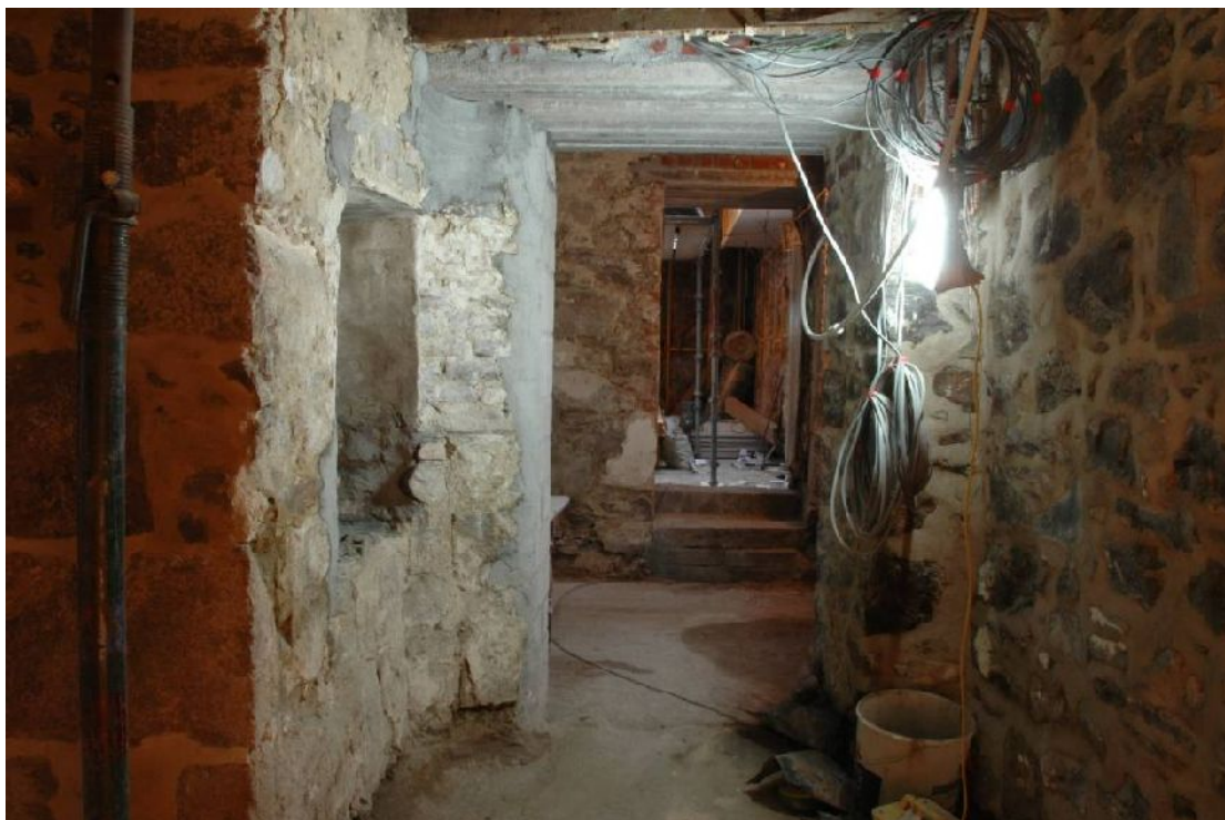
Illus 62 Looking towards the Pend from the Dining Room showing passage after D9 removed.
