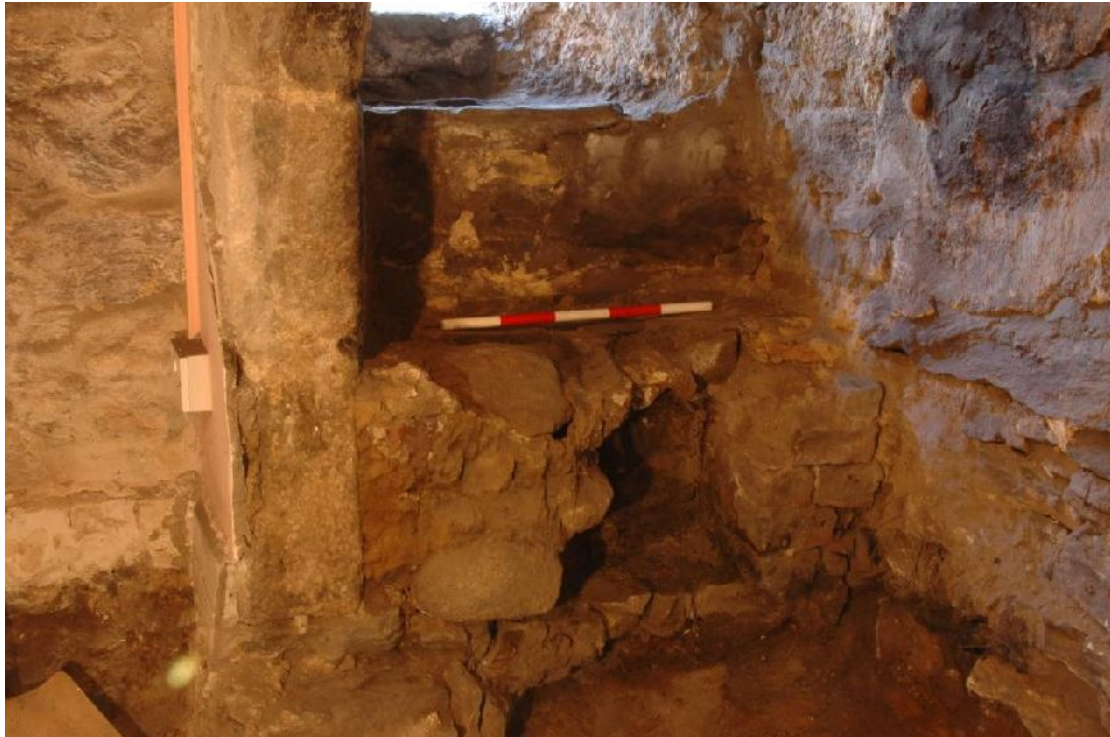
Illus 54 Window W5 from inside showing possible seat, after removal of rubble
