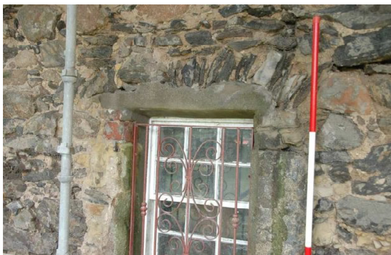
Illus 22 Window W8 after harling removed 2013. Relieving arch visible.
