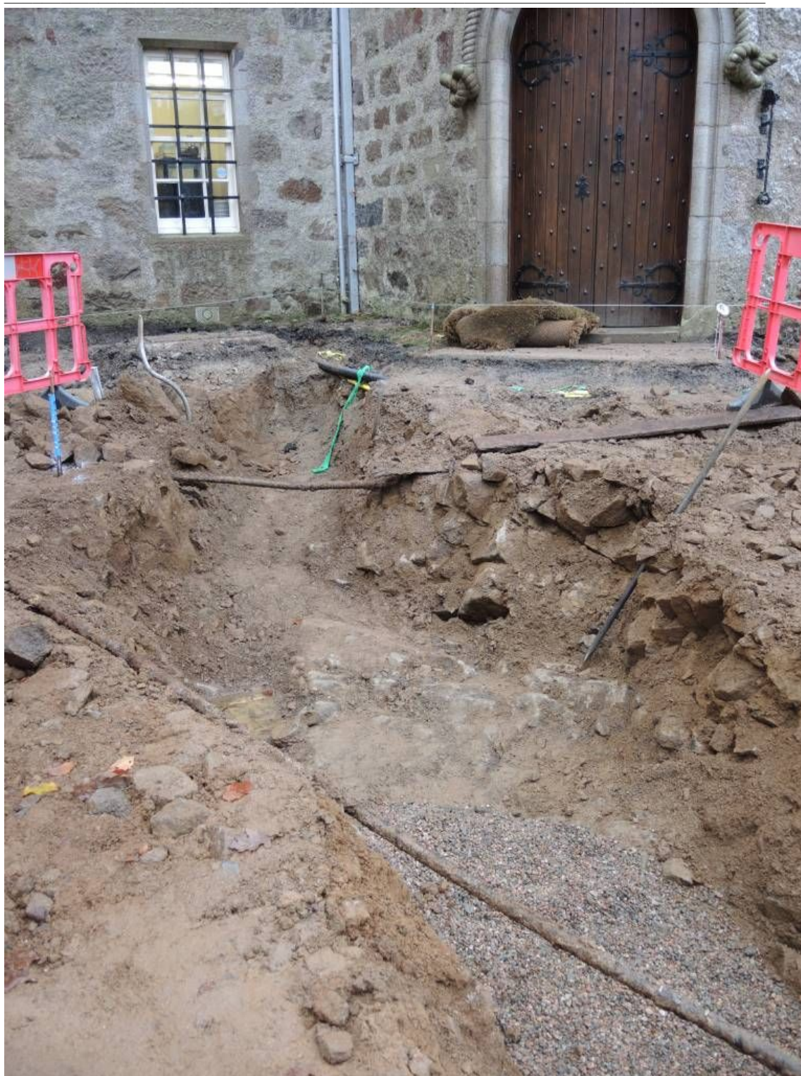
Illus 51 SE area of courtyard with natural cut for inserting drains. Note bedrock.
