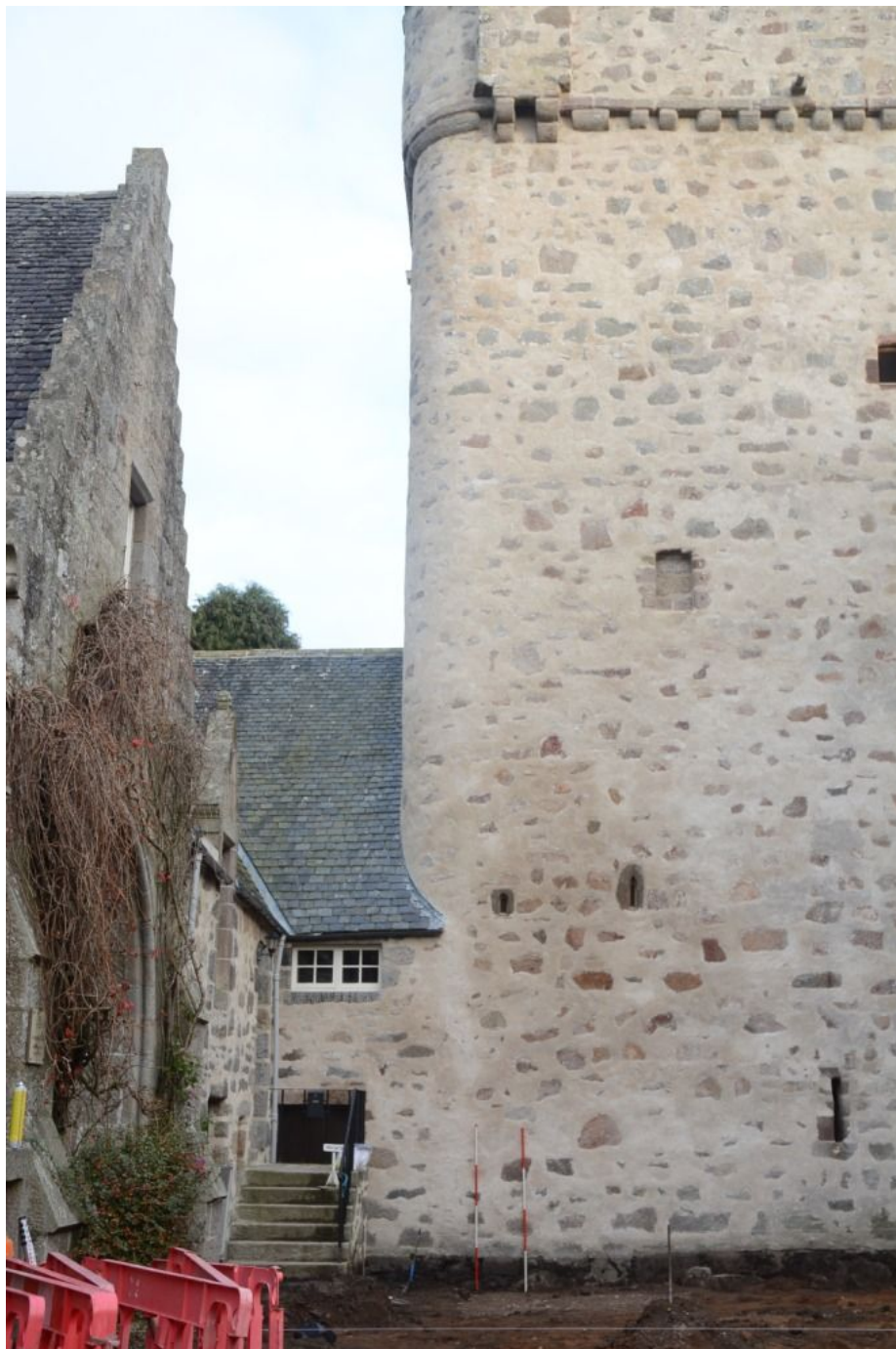
Illus 52 W wall of tower. The two vertical ranging rods flank the possible blocking of drain outlet from intra-mural garderobe
