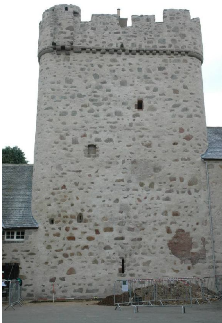
Illus 7 View of W wall of tower with garderobe at NW/ Ranging rods mark position of cess pit in Area 1.
