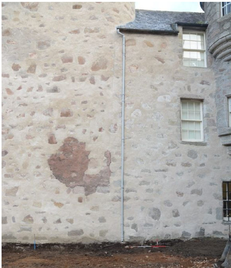
Illus 58 Cross range W wall. Ranging rod indicates the position of exposed foundation.
