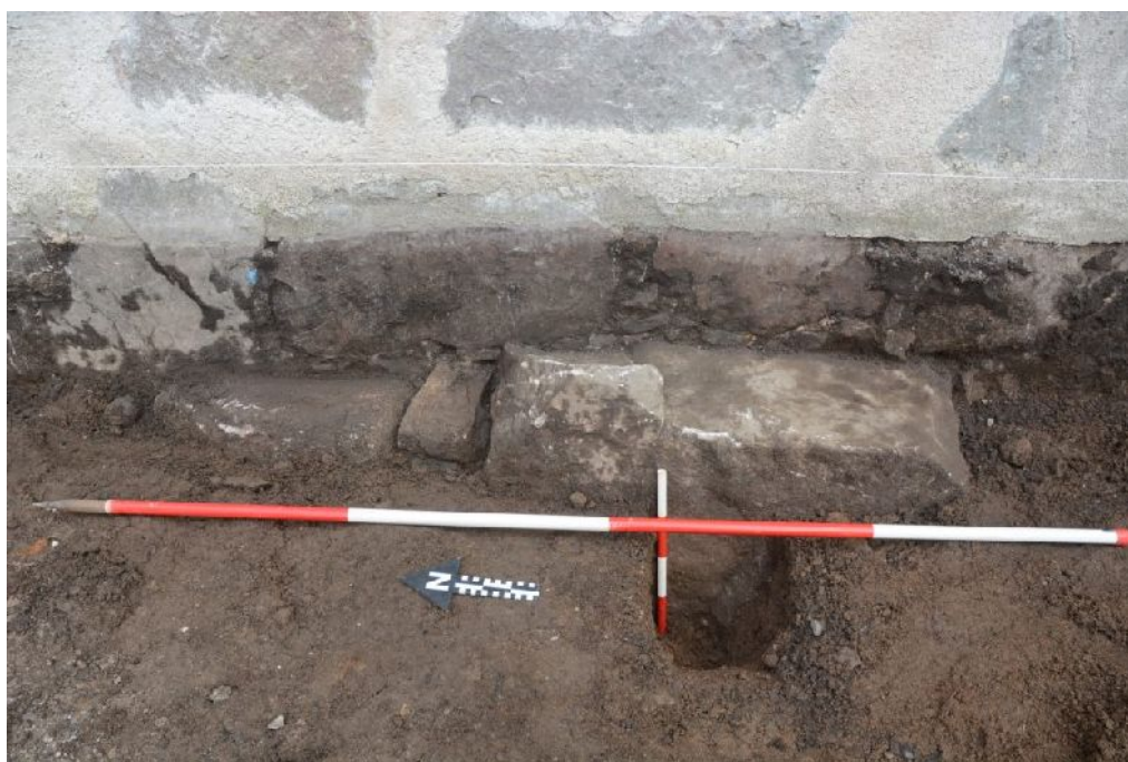
Illus 56 Tower W wall. Detail of projecting natural boulders incorporated into base of wall.
