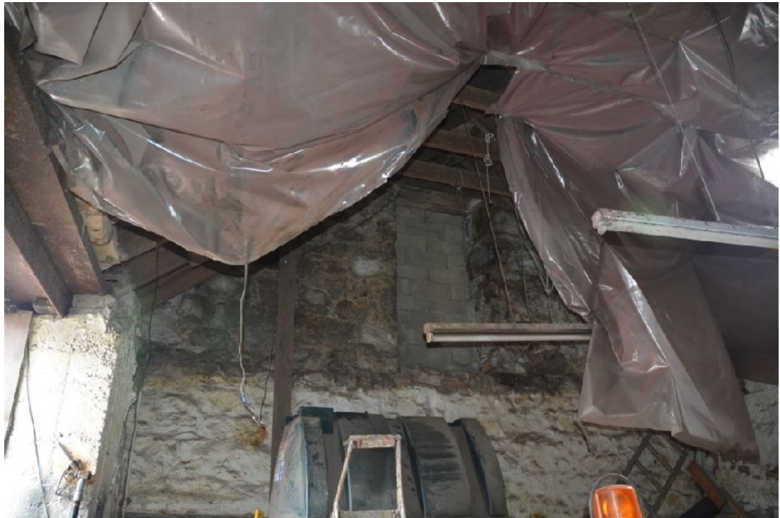
Illus 9 Building 2. S steading. Internal view of internal wall and part of loft at E end (Photo 2)
