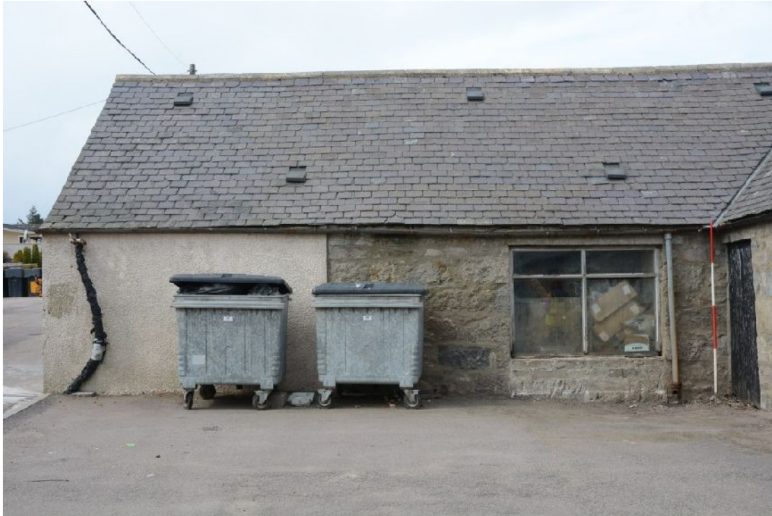
Illus 13 Building 3. N steading. E wall of W range. Shows window W1 built in earlier opening. (Photo 12)
