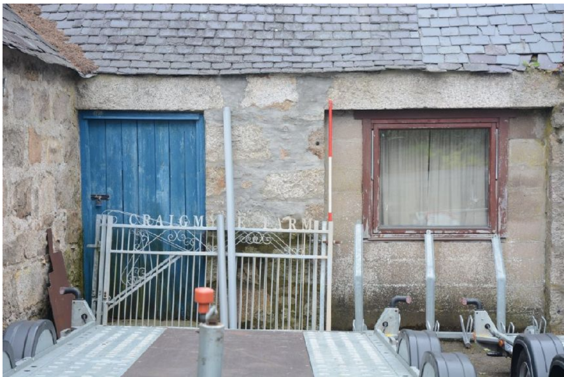
Illus 11 N Range, S wall. Door D3 and D4 with W1 inserted.
