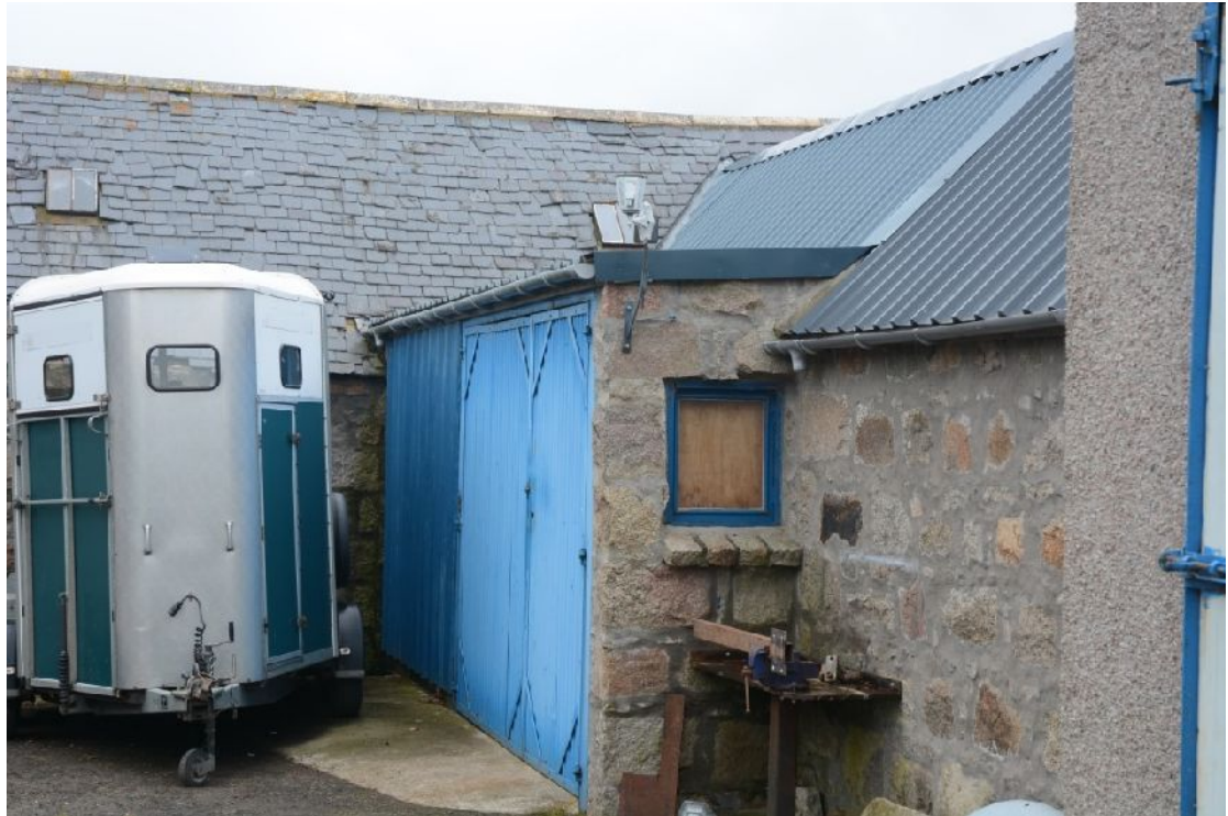
Illus 18 E Range Building 2.W wall showing flat-roofed extension, D5 and W2
