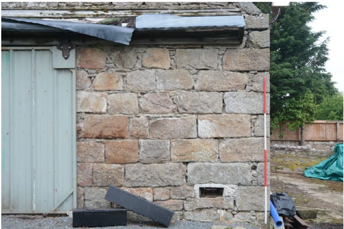
Illus 9 Detail of E gable of N range. Note blockwork. Concrete blocking at base of wall appeared to be modern knock-through.
