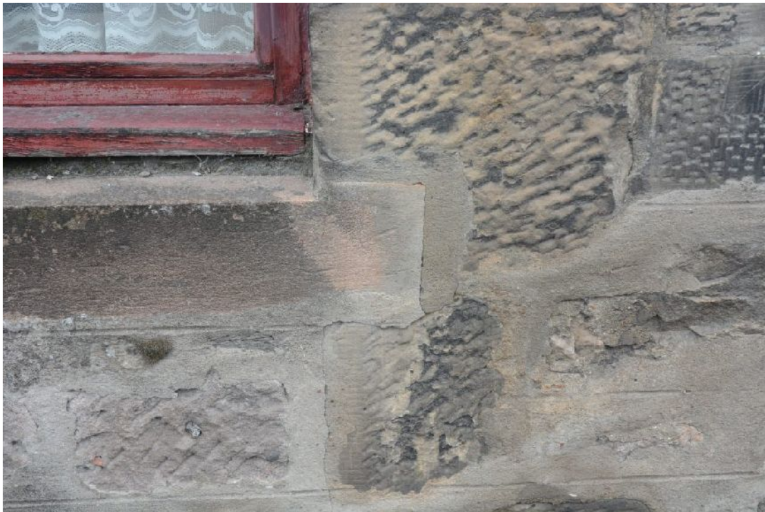
Illus 13 Detail of bottom RHS of W2 showing new sill breaking across rybats of earlier door.
