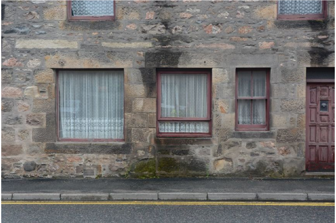
Illus 12 W elevation from LHS: W1, W2 with blocking below and W3
