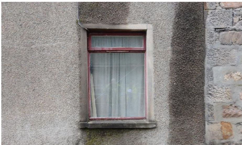
Illus 5 Window W10 with concrete surround. Note on RHS junction between the earlier stone building and the later concrete building.
