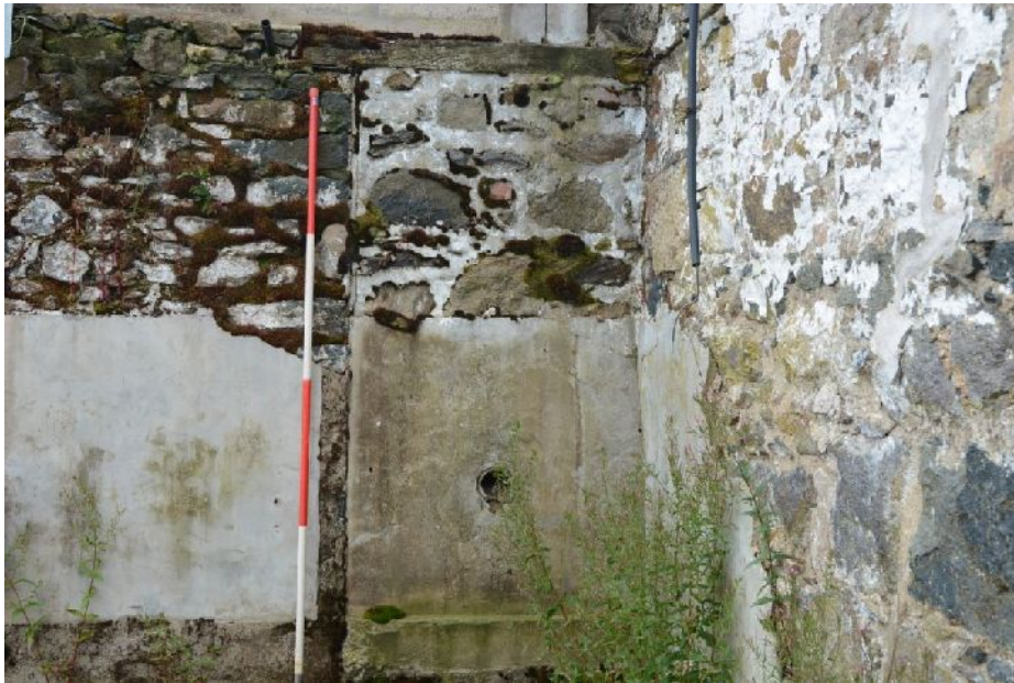
Illus 14 B3. Blocked door D17 showing wooden lintel to interior of B3.
