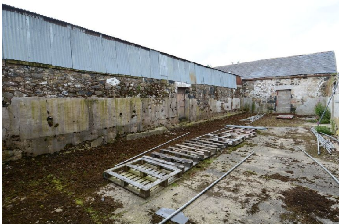
Illus 15 B3 interior looking W to wall of B2. Note scars of tied cow stalls on wall to LHS
