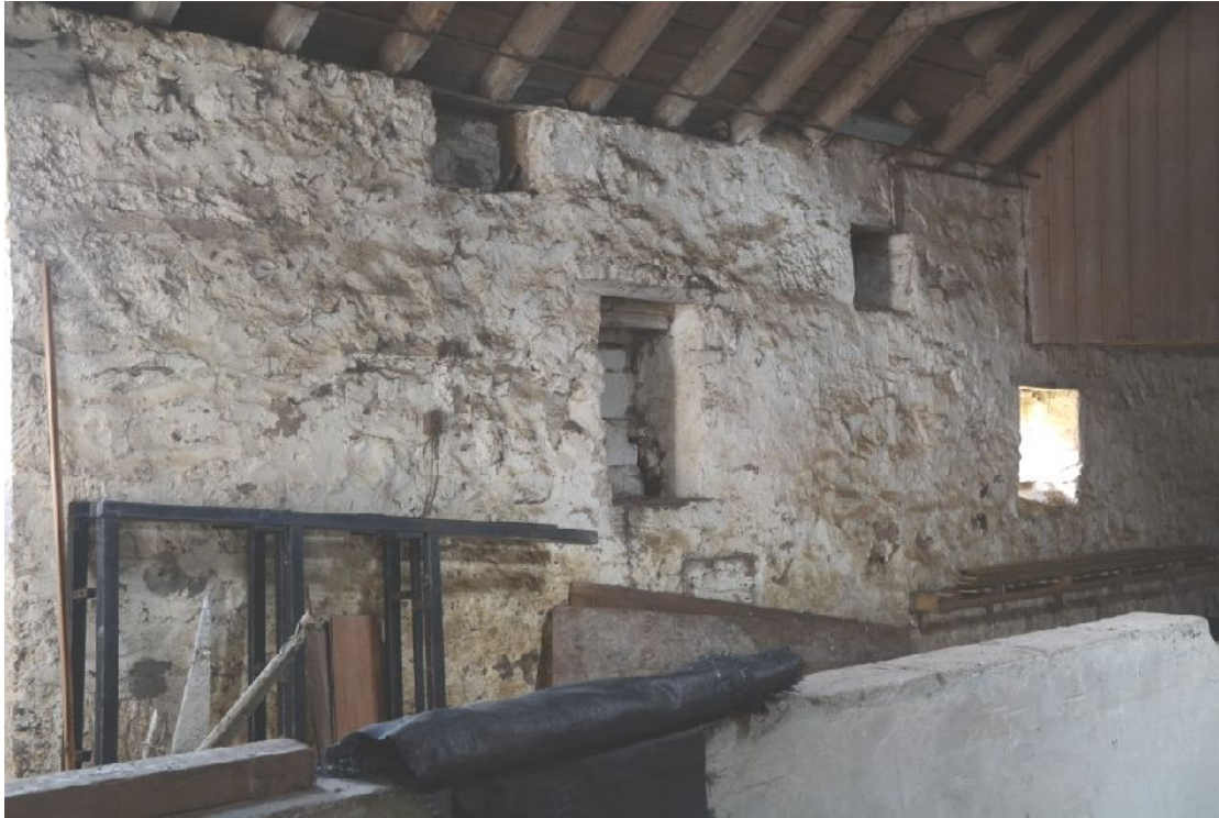
Illus 11 Inside of W wall of B2. Openings associated with mill From LHS to RHS: F5 (at top- not visible externally), F1, F2, F3, F4 (with light through).
