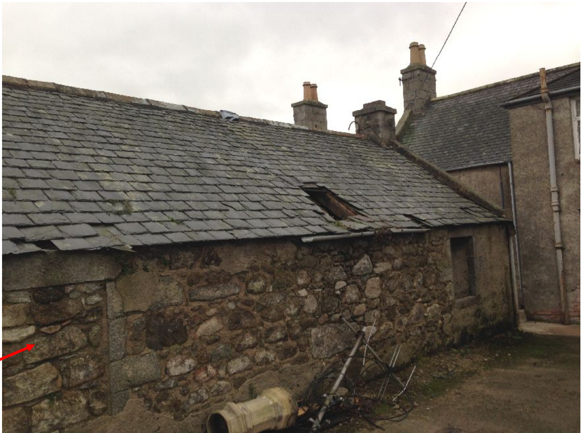
Illus 10 NW wall looking W. Arrow indicates D3. Photograph prior to partial demolition (Photograph courtesy of Baxter design)
