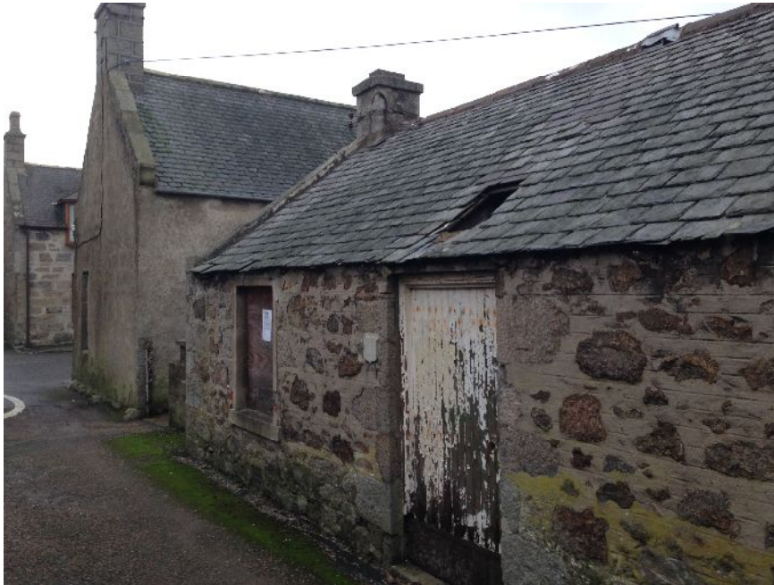
Illus 2 Cottage looking towards High Street prior to partial demolition (Photograph courtesy of Baxter design)
