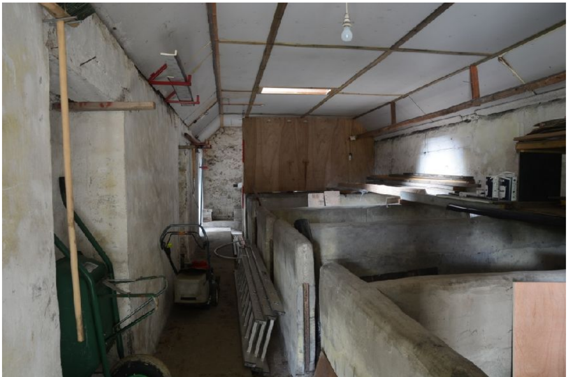
Illus 12 Looking W through room B showing raised concrete floor and pigs stalls.
