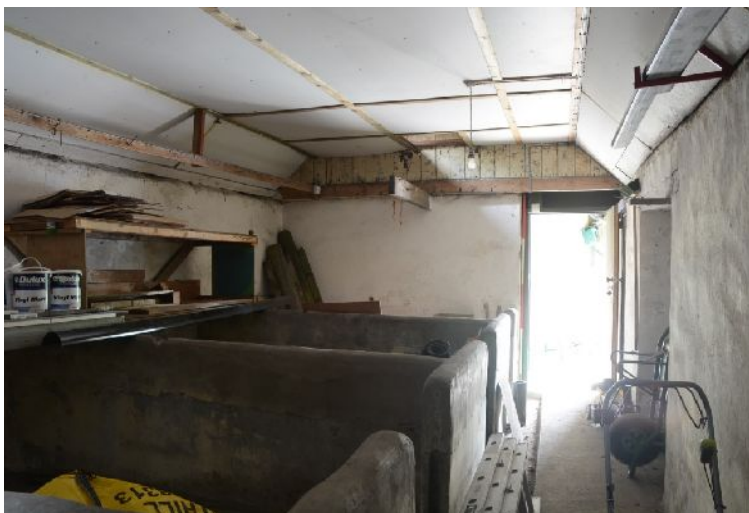
Illus 10 Looking E from room B towards room A. Shows base of the timber loft wall and position of projecting timber.
